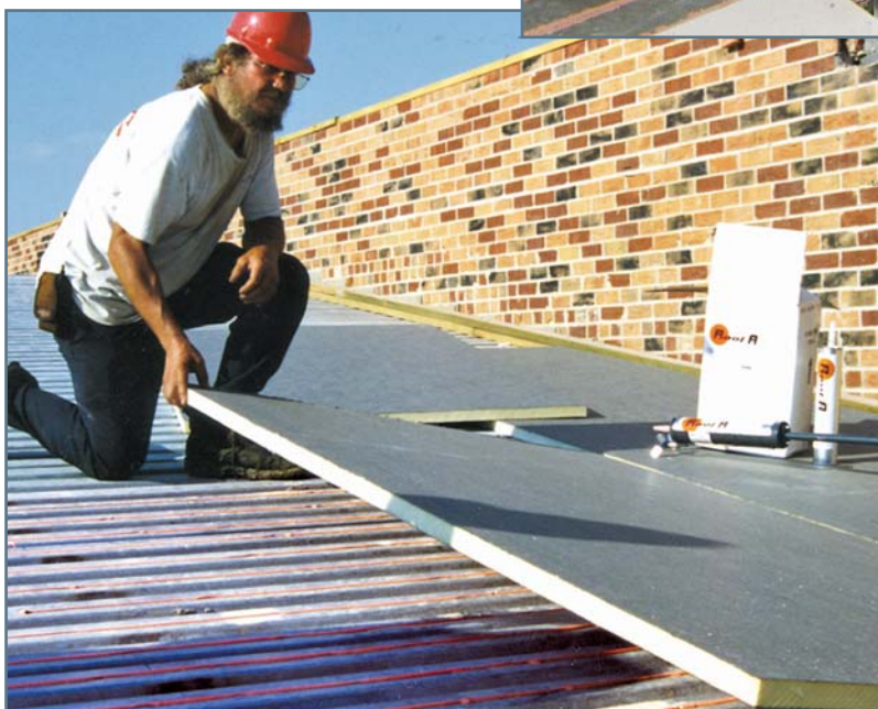
Photo 4 – New thermosetting foam and moisture-cure adhesives can make the roof safer while providing superior wind uplift performance compared to mechanical fasteners.
