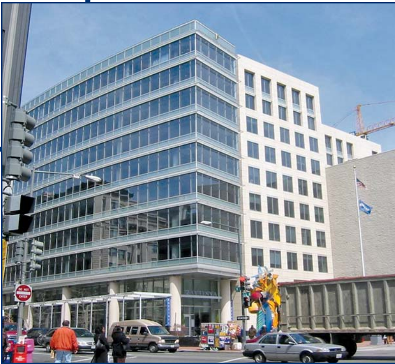
Photo 4 – The precast concrete wall panels and spandrel glass in the curtain wall are barrier systems.
