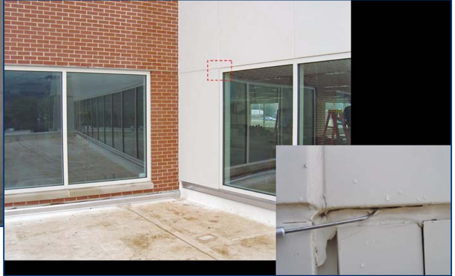
Photo 11 – A sealant breach (inset) was the leak source within this multicomponent wall assembly.
