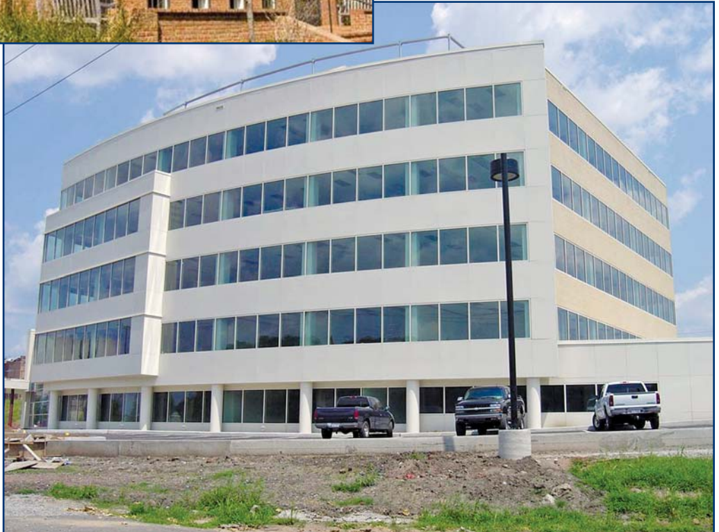
Photo 3 – This wall system incorporates a drained window assembly in a continuous band.
