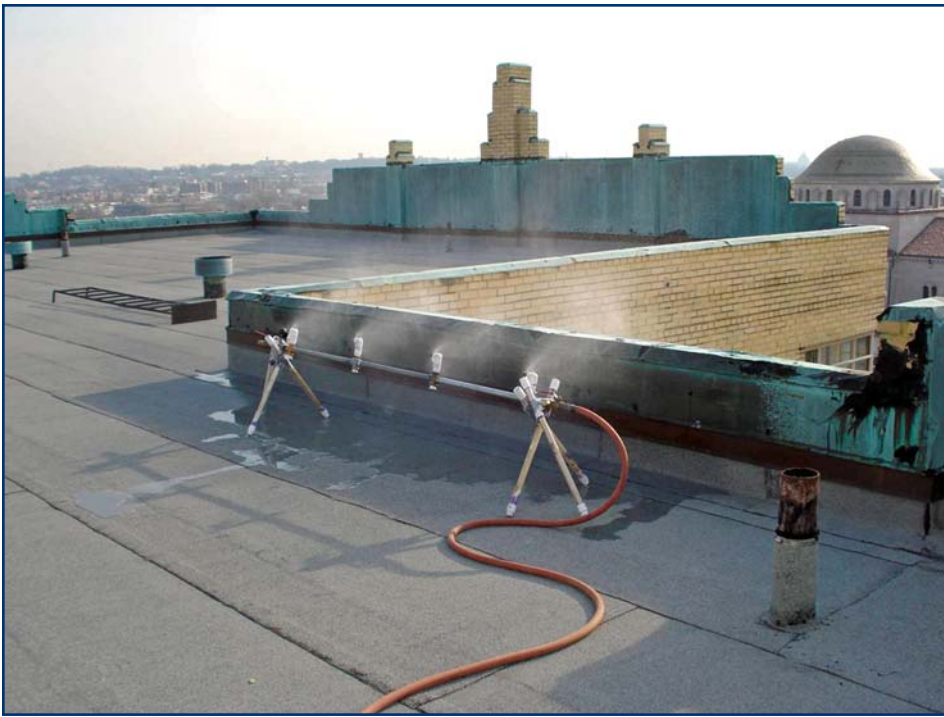
Photo 14 – A spray rack in use to test the interior side of a parapet wall.
