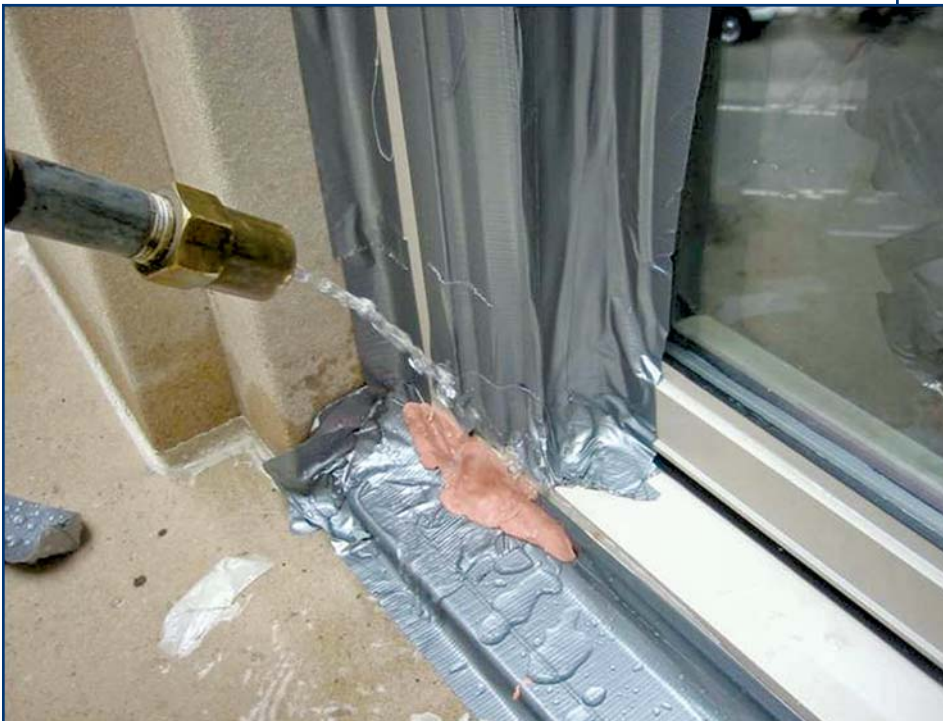
Photo 13 – Duct tape and putty are used to mask joints within a window to isolate a leak source.
