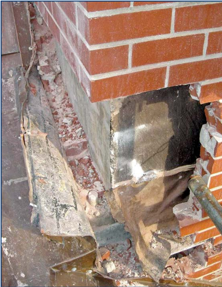
Photo 16 – Exterior inspection shows an opening exposing flashing deficiencies in a masonry cavity wall.
