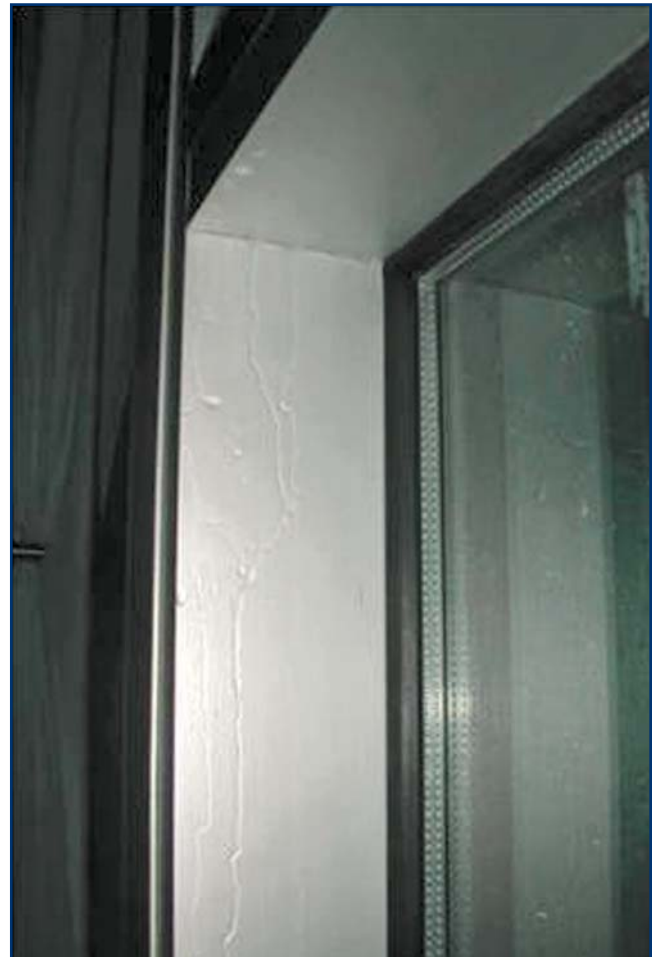
Photo 15 – Moisture-sensitive paper indicating a leak at the window interior perimeter.
