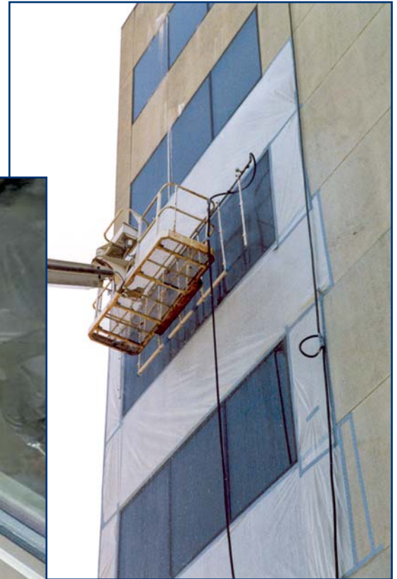
Photo 12 – Plastic sheeting is used to isolate the window system from the wall panels during testing.
