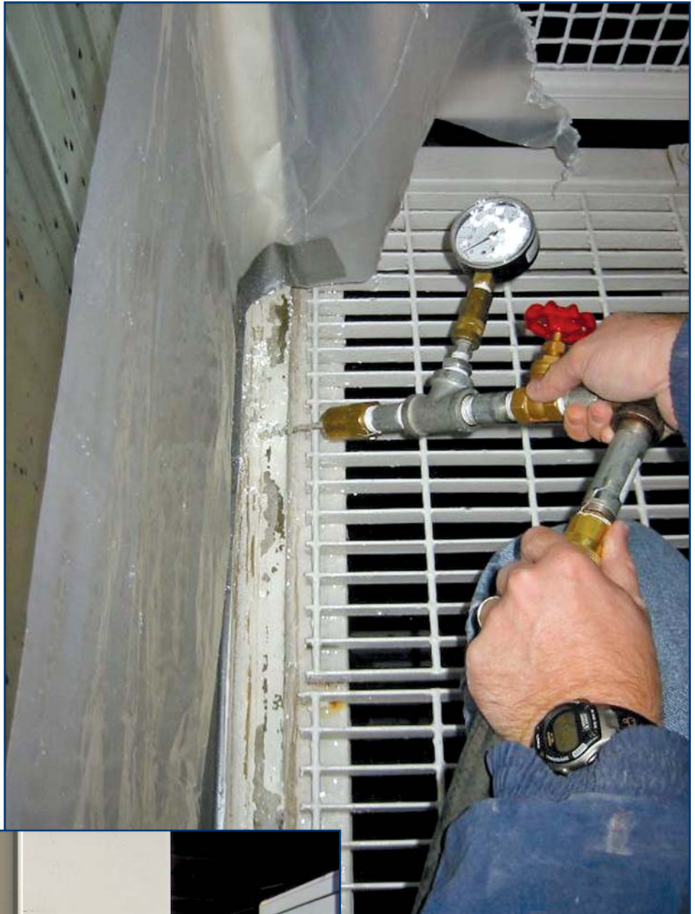
Photo 7 – Nozzle testing in progress; note the minimal flow rate to isolate a specific leak source.
