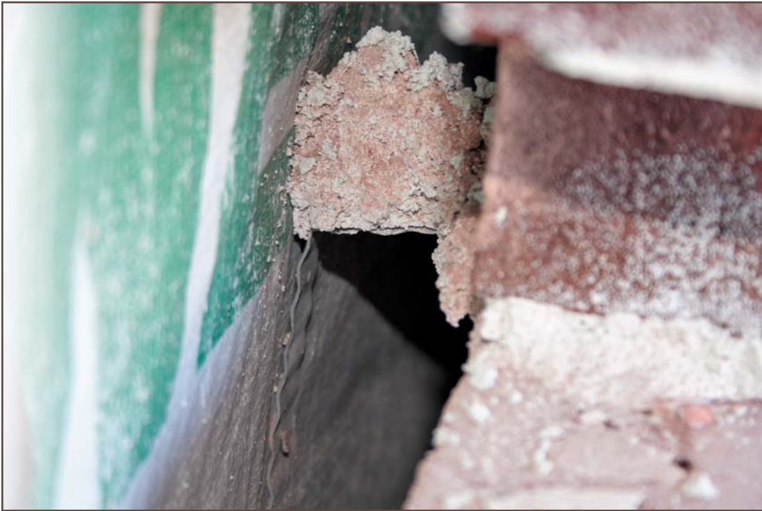
Photo 1 – Mortar droppings collect on top of metal brick ties and bridge across the 1-inch air space, coming into direct contact with a highly permeable weather-resistant membrane.
