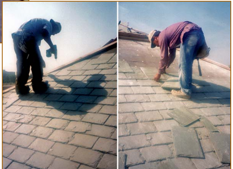
Figure 18 – It is a mistake to walk on a slate roof during installation.
