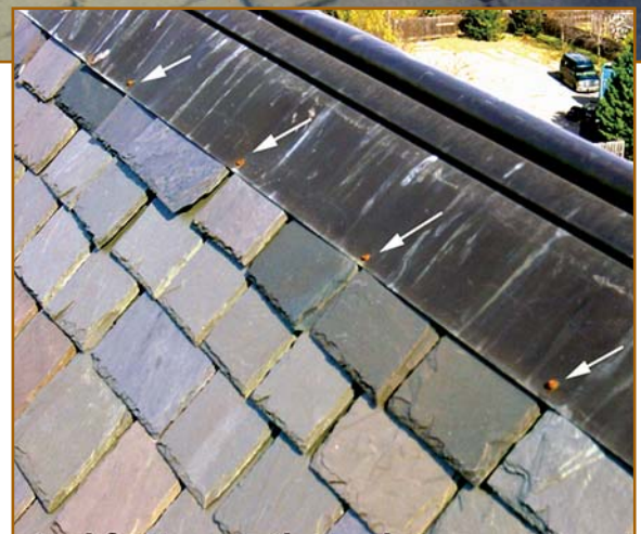
Figure 28 – Metal fasteners should always be compatible with the metal they are fastening. Steel fasteners on copper, as shown, will deteriorate.
