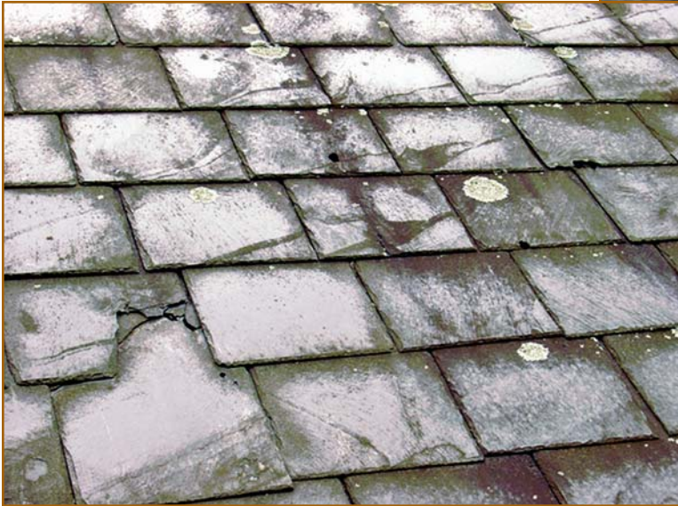
Figure 13 – Each slate side-butt should be staggered so as to break the course below down the center. Instead, these slates were butted directly over the underlying slating nails, ensuring leakage.
