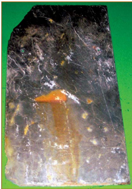
Figure 2 – This Spanish black slate leached rust stains down the new slate roof. This photo shows the slate after only one year on the roof.
