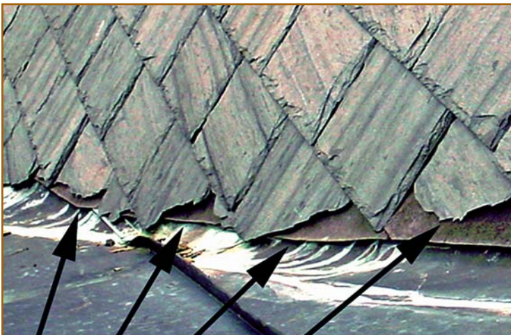
Figure 33 – Slate roofing requires the correct tools to do the job right. There is no excuse for the sort of work shown here.
