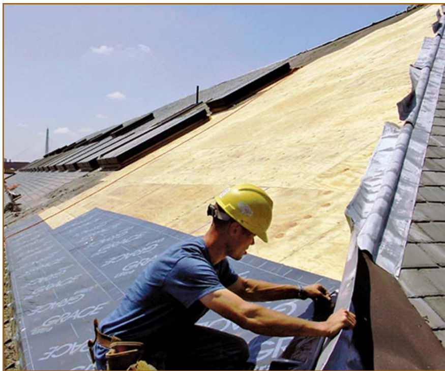
Figure 4 - Traditional slate roofing systems, despite their incredibly successful performance, are being largely abandoned in favor of plywood roofs with peel-and-stick underlayments.
