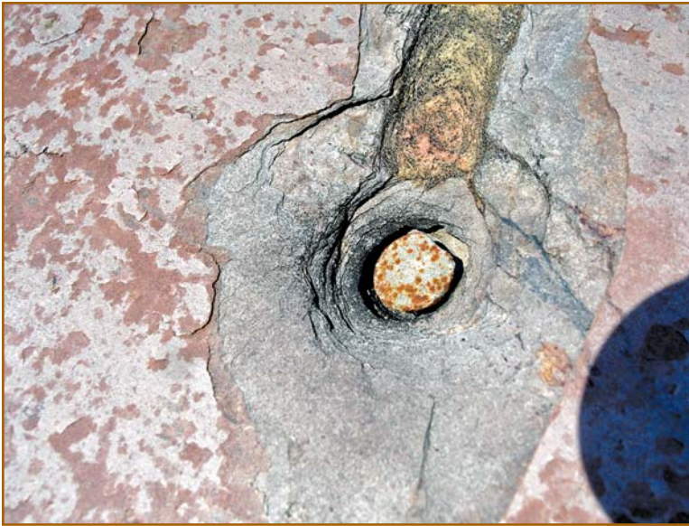
Figure 15 – A protruding nailhead can eventually wear a hole in the overlying slate.
