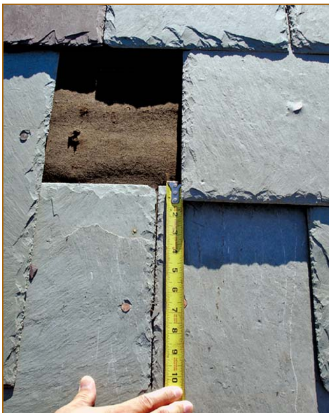
Figure 10 – This is an example of inadequate headlap on a shopping center roof in Louisiana.
