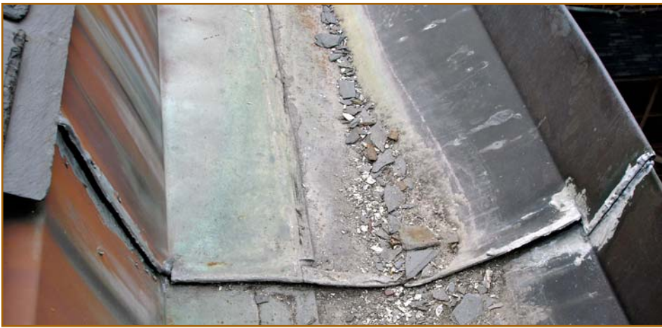
Figure 25 – This is a perfect example of a new built-in gutter showing failed solder joints because not a single expansion joint was installed in the gutter system.
