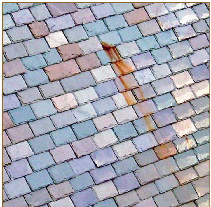
Figure 3 – Even domestic slates can rust. These Vermont slates on a high-rise apartment were poor in quality and should have been screened for pyrite inclusions.
