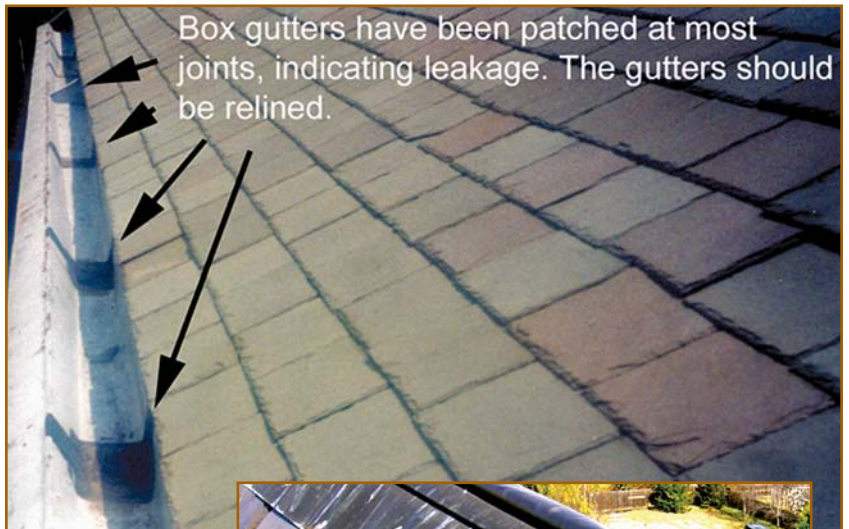
Figure 26 (above) – Box gutters require expansion joints; otherwise, the solder joints will crack under pressure. This is evidenced by solder joints that have been covered by roof cement, a common sight on box gutters, both new and old.
