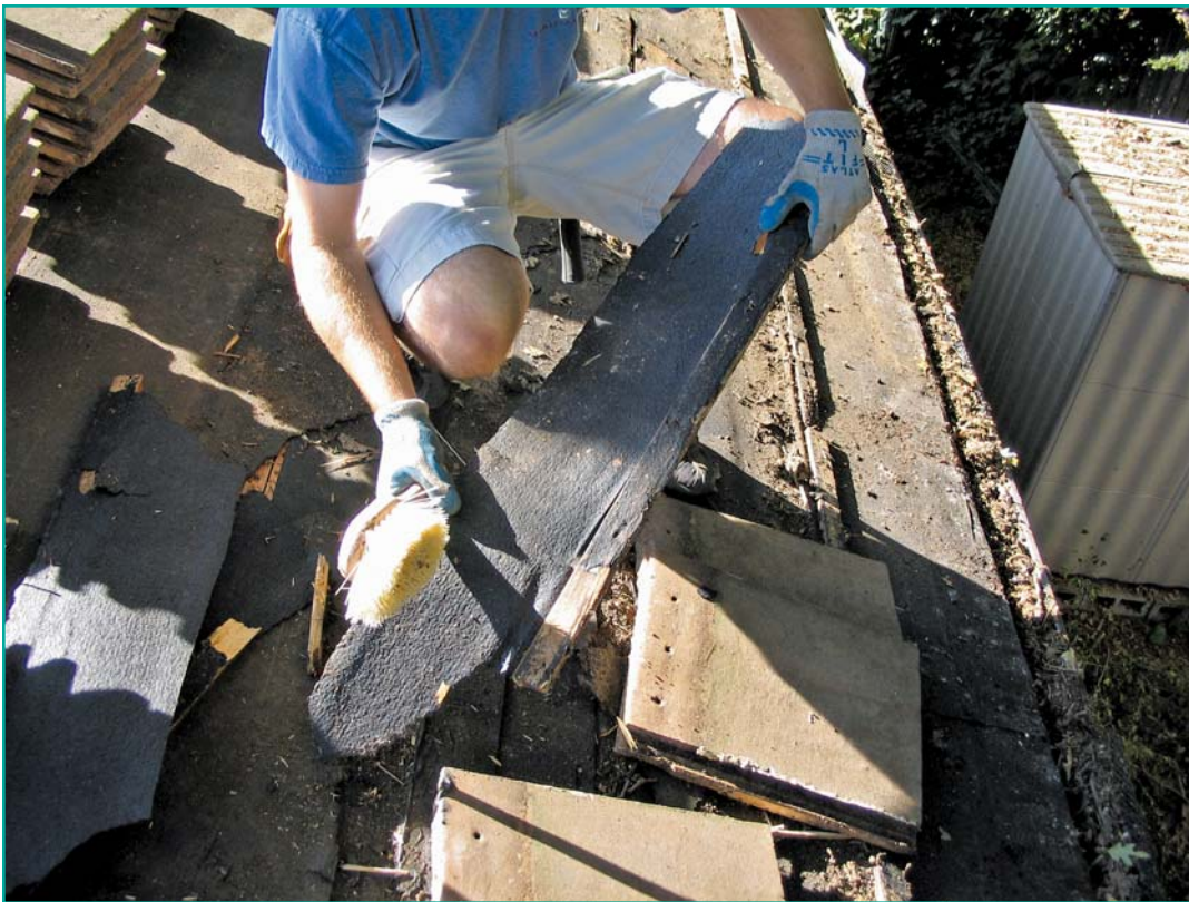
Figure 5 – Trapped moisture gradually destroys most underlayments, resulting in roof leaks.
