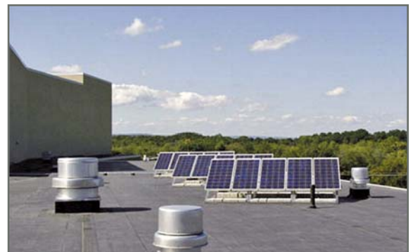
Figure 1 - Crystalline-silicon array on a Voorheesville, NY, school. Photo courtesy of New York State Energy Research & Development Authority.
