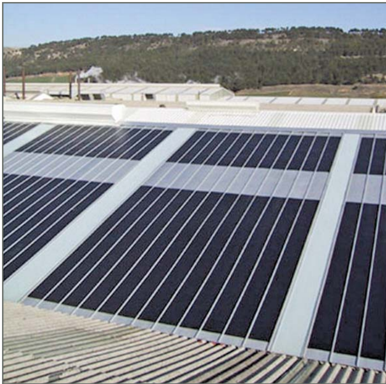
Figure 3 - Uni-Solar metal panels with thin-film photovoltaics.
