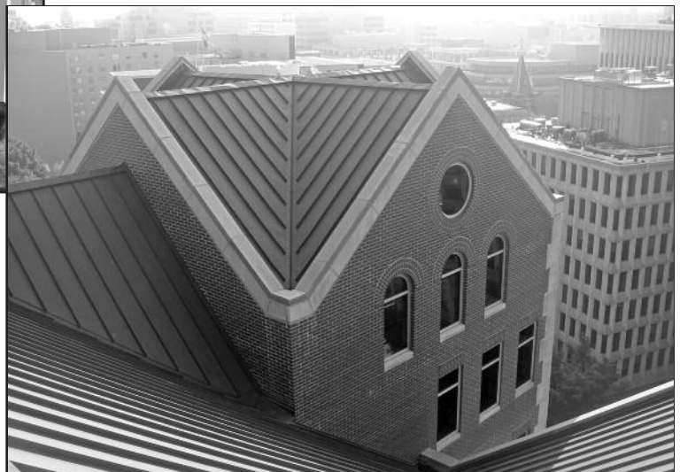
Figure 7 – Copper roofing improperly terminated at raked masonry rising wall.
