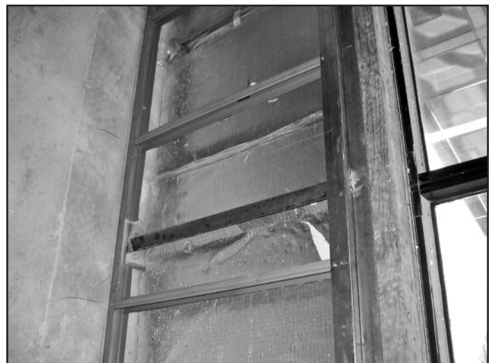
Photo 12 – Installation of supplementary steel framing at the interior side of a concrete masonry backup wall.
