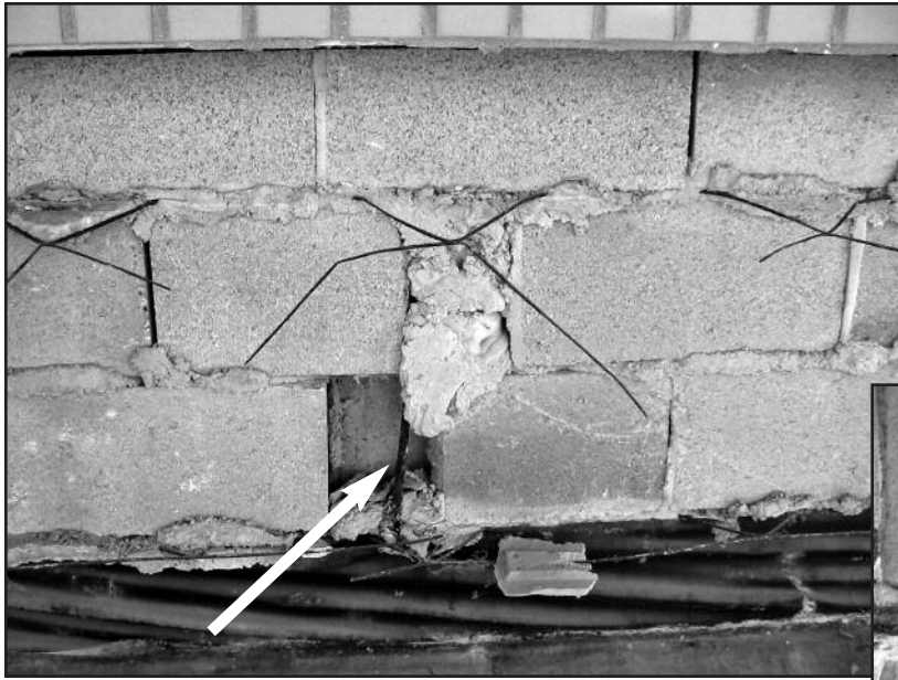
Photo 8 – Corroded steel reinforcement (arrow) and truss reinforcement in a concrete masonry backup wall. Also note incompletely filled head joints, exposed reinforcement, and lack of waterproofing membrane on backup.
