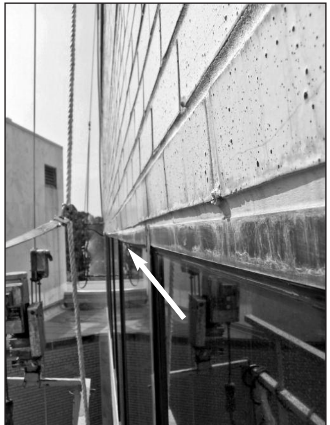
Photo 5 - Window sagging (arrow) as result of the downward deflection of the shelf angle.
