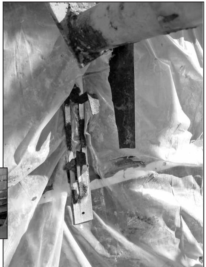
Photo 7 – Corroded adjustable brick tie over plastic sheathing. Note brick tie is attached through plastic sheathing and exterior sheathing to steel stud.
