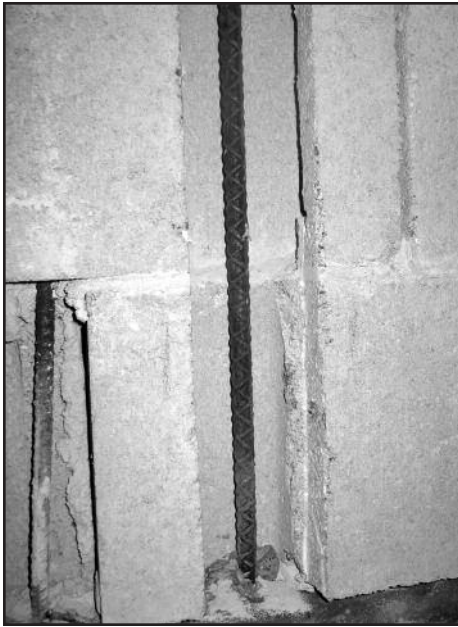
Photo 10 – Installation of steel reinforcement into cavities cut into the concrete masonry backup wall as part of remedial work.
