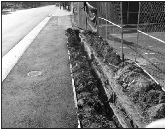
Excavation of the soil behind the wood lagging revealed that once the wood gets wet, it swells, bends, and twists, especially if there are voids between the soil and wood.
