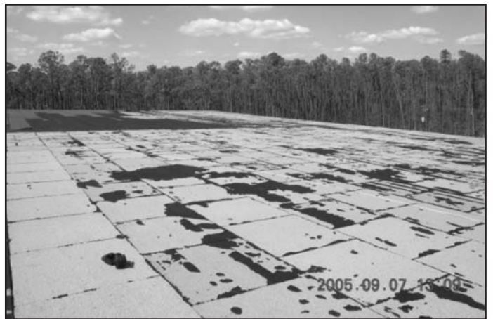
Figure 6 – Membrane peeled off the insulation (photo courtesy of RICOWI Inc.).
