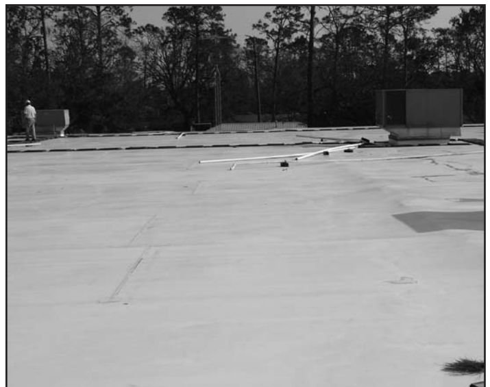
Figure 4 – Adhered single-ply membrane after Hurricane Ivan. (Photo courtesy of RICOWI Inc.)
