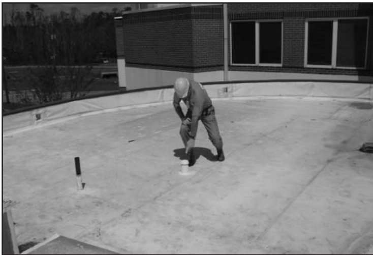
Figure 3 – Mechanically fastened thermoplastic single-ply membrane after Hurricane Katrina. (Photo courtesy of RICOWI Inc.)
