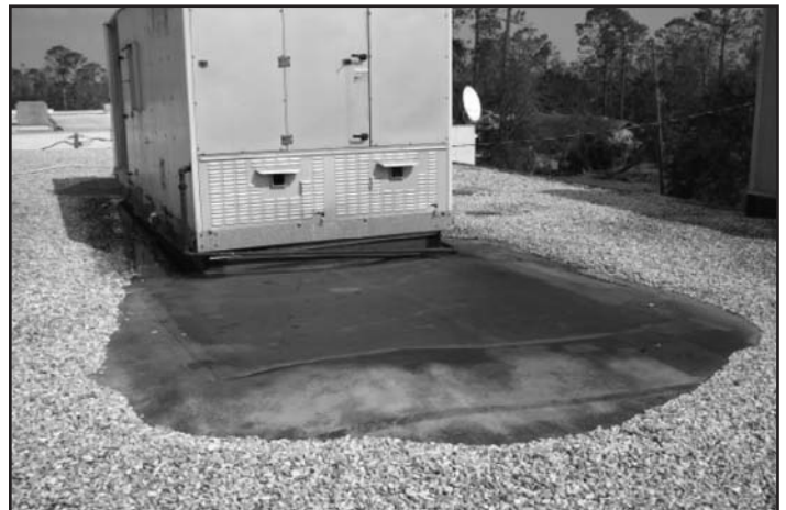
Figure 2 – Example of stone scour that can occur in areas of localized high wind loads (photo courtesy of RICOWI Inc.).
