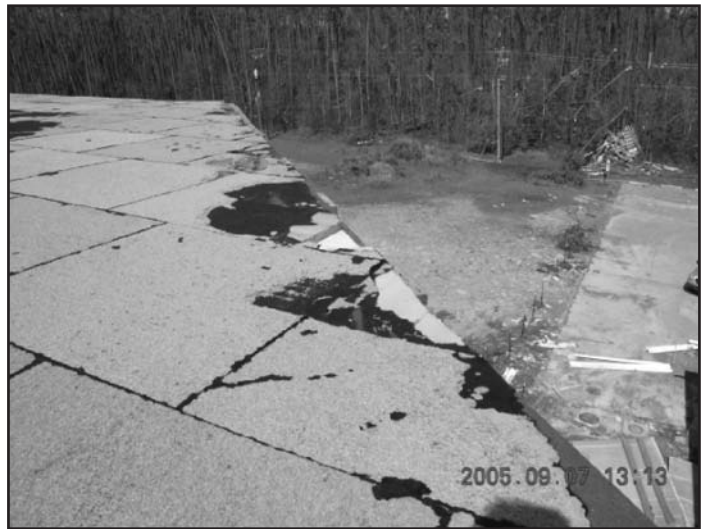
Figure 5 – Edge metal attachment lost (photo courtesy of RICOWI Inc.).
