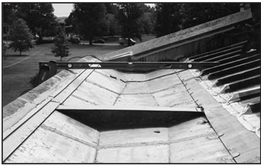
Figure 2 – The outside edge of this built-in gutter liner is let into a reglet in the limestone coping stone. Compare this image to Revere's detail shown in Figure 7. Note, too, that the expansion joint is below the high water line of the gutter (compare to Figure 15).
