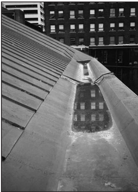
Figure 4 – Trough-level, membrane expansion joint in a large, built-in gutter. Three expansion joints have been installed atop one another, creating a dam. The gutter outlet is located in the distance, near the gutter-end wall.
