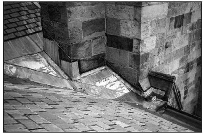
Figure 5 – This lead-coated, copper built-in gutter has been re-lined with an EPDM membrane. The exposed edge of the membrane bucks water at the valley. Note, too, all of the tight inside and outside corners the membrane must accommodate.
