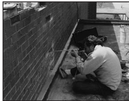
Figure 5 – Performing a boroscope analysis to view wall cavity and related back-up wall components.
