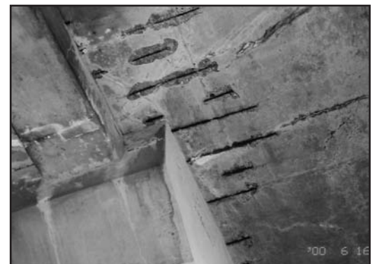
Figure 7 – Steel reinforcement corrosion resulting from high chlorides and presence of carbonization.
