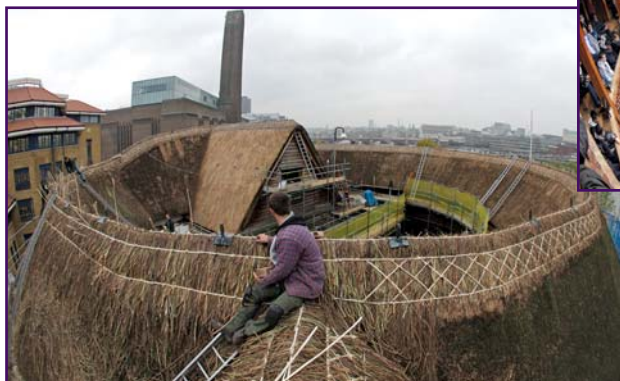
Ridding nearing completion. Left-hand side of stage roof newly thatched. Photo © Nathan Harrison.
