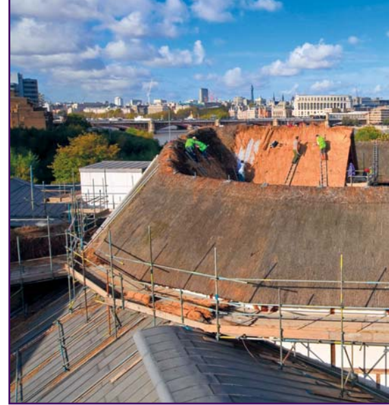
Workers can be seen on the interior roof. St. Paul's Cathedral is on the far right. Photo by Pawel Libera.
