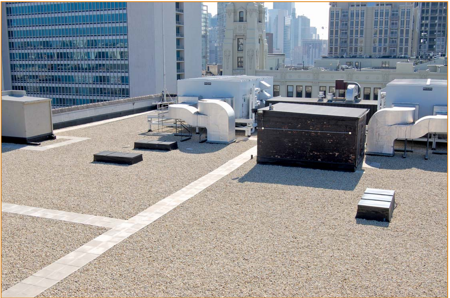
Photo 1 – In colder climate regions, such as Chicago, IL, construction-generated moisture may be detected in the form of drips inside the building after the first freeze/thaw cycle. These drips are sometimes misinterpreted as roof leaks. The ballasted EPDM roof shown here at 600 West in Chicago did not experience any moisture-related problems after construction. (Photo courtesy of Tom Hutchinson, Hutchinson Design Group Ltd., Chicago, IL.)
