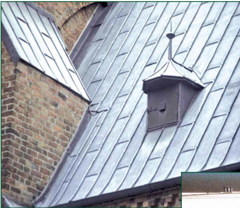
Figures 11 and 12 – In the early days of metal roofing, pan lengths were short, so thermal movement never accumulated. As the “unbroken length” of panels increases, so does the dimensional gain or loss due to differences in surface temperature.
