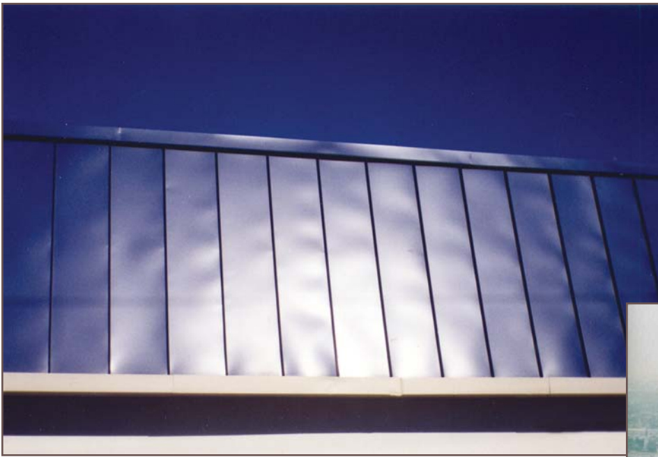
Figure 2 – Almost any metal roof will exhibit some oil canning in direct angles of sunlight. The displeased party should exercise patience, as the eventual patina will obscure most of the oil canning.
