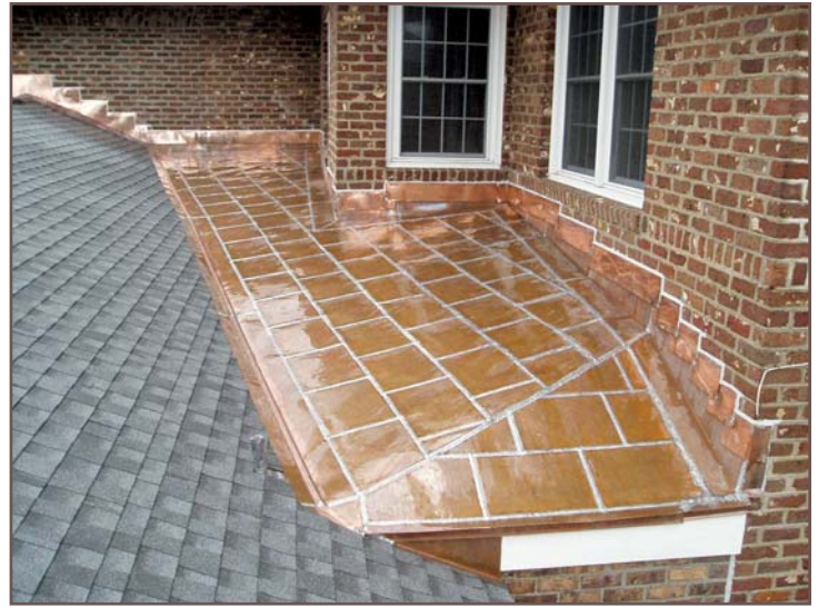
Figure 4 – Especially for low-slope, flat-seamed copper, the time-honored skill of soldering is absolutely central to satisfactory performance. (Photo courtesy of Christopher Waites, ADC Engineering, Inc.)
