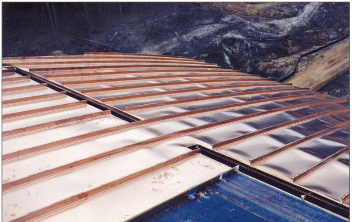
Figure 1 – Introducing flat pans onto a curved surface can and will produce surface undulations. On curves having a long radius, the susceptibility is lower.
