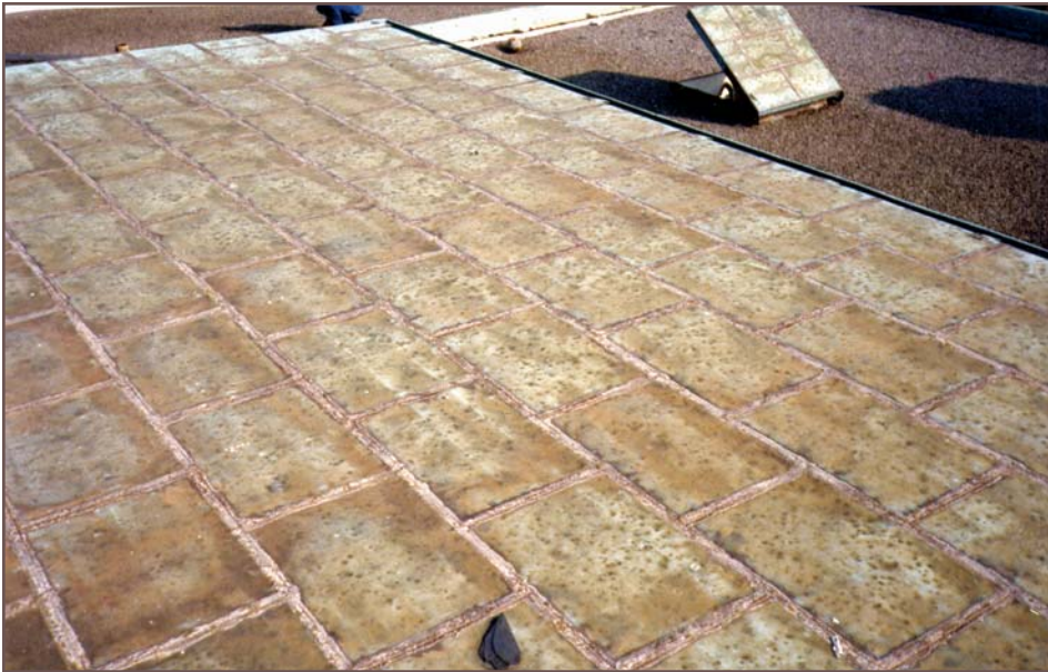
Figure 5 – Minor hail indentations in a copper roof do not compromise water-shedding capability (or service life expectancy). If eventual hail dents in copper cladding will be considered analogous to dents in the fender of an automobile, an alternative covering should be considered.
