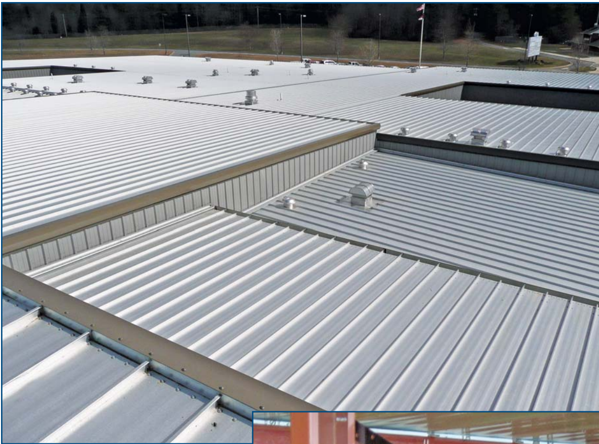
Photo 3 – Low-sloped, unpainted metal roof on a high school in central North Carolina.
