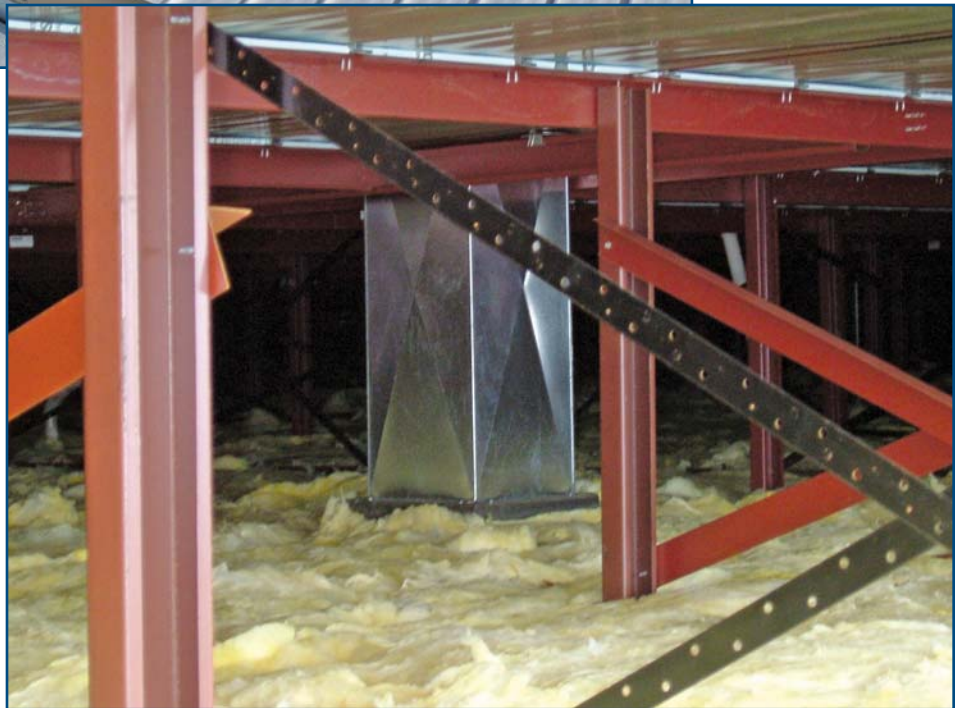
Photo 4 – The open cavity between this new metal roof and the roof insulation needs to be ventilated.
