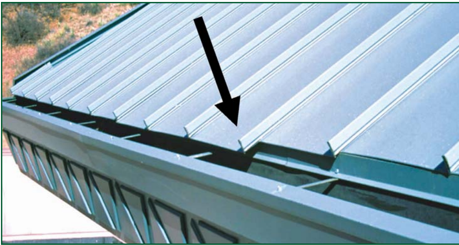
Figure 7 – If a panel is not “fixed” at some location, gravity or “drag loads” can pull it down the slope of the roof.
