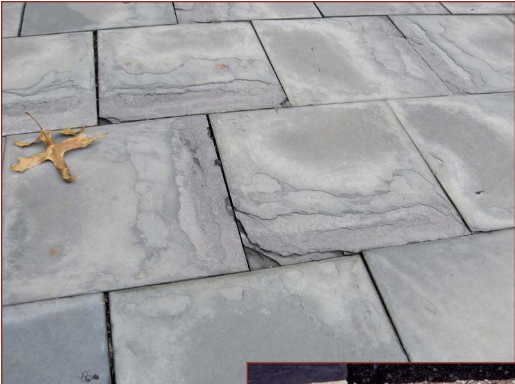
Photo 1 – Freeze-thaw damage to stone pavers.
