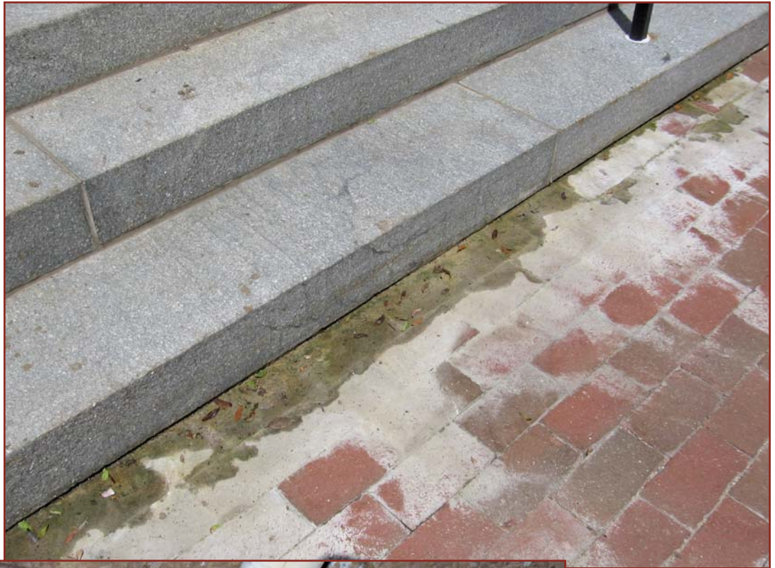
Photo 4 – Efflorescence on brick pavers at the base of stairs.
