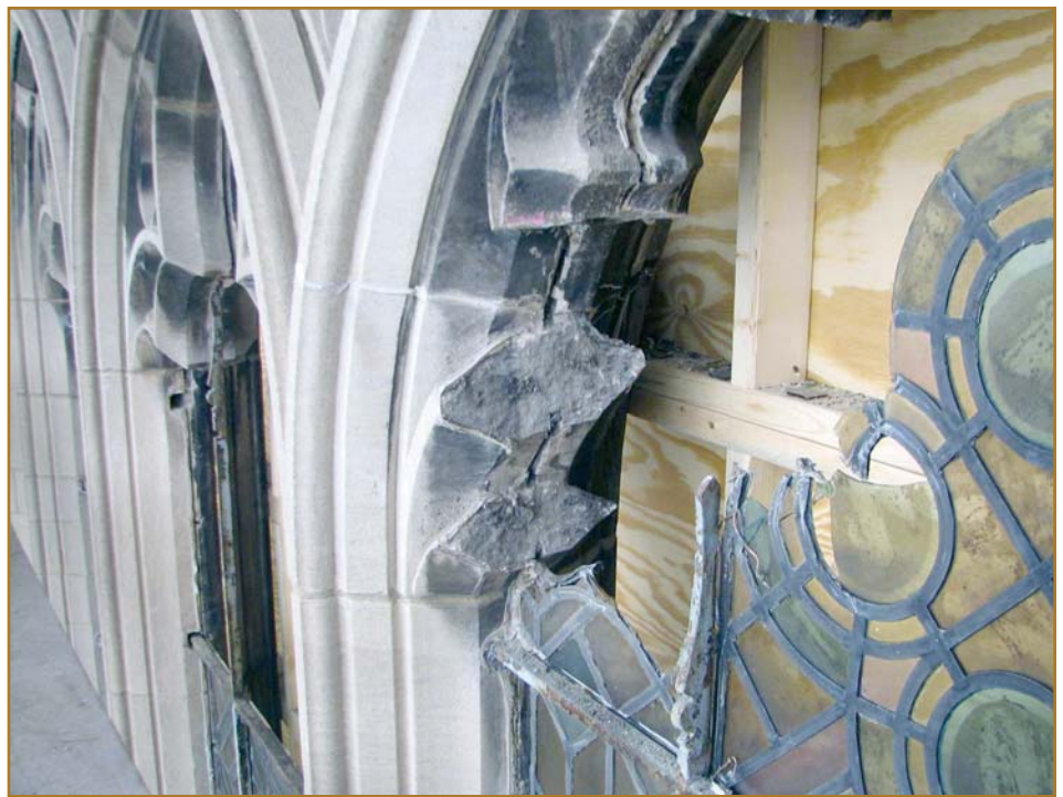
Photo 12 – At some locations, the stained glass and exterior support framing provided supplemental support to damaged stone tracery.
