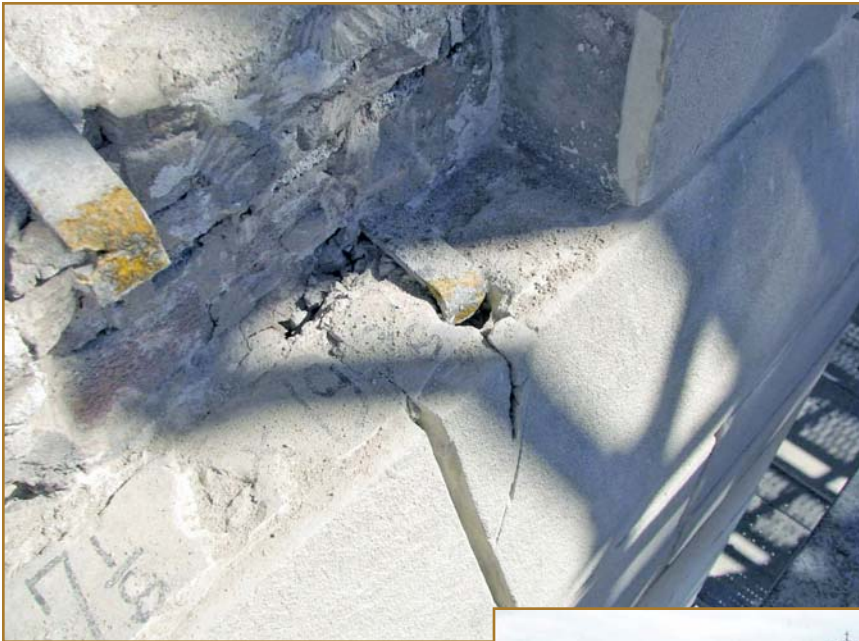
Photo 8 – Typical stone distress resulting from corroded steel strap and/or the open cell (receiver) in the stone subjected to freeze/thaw damages.
