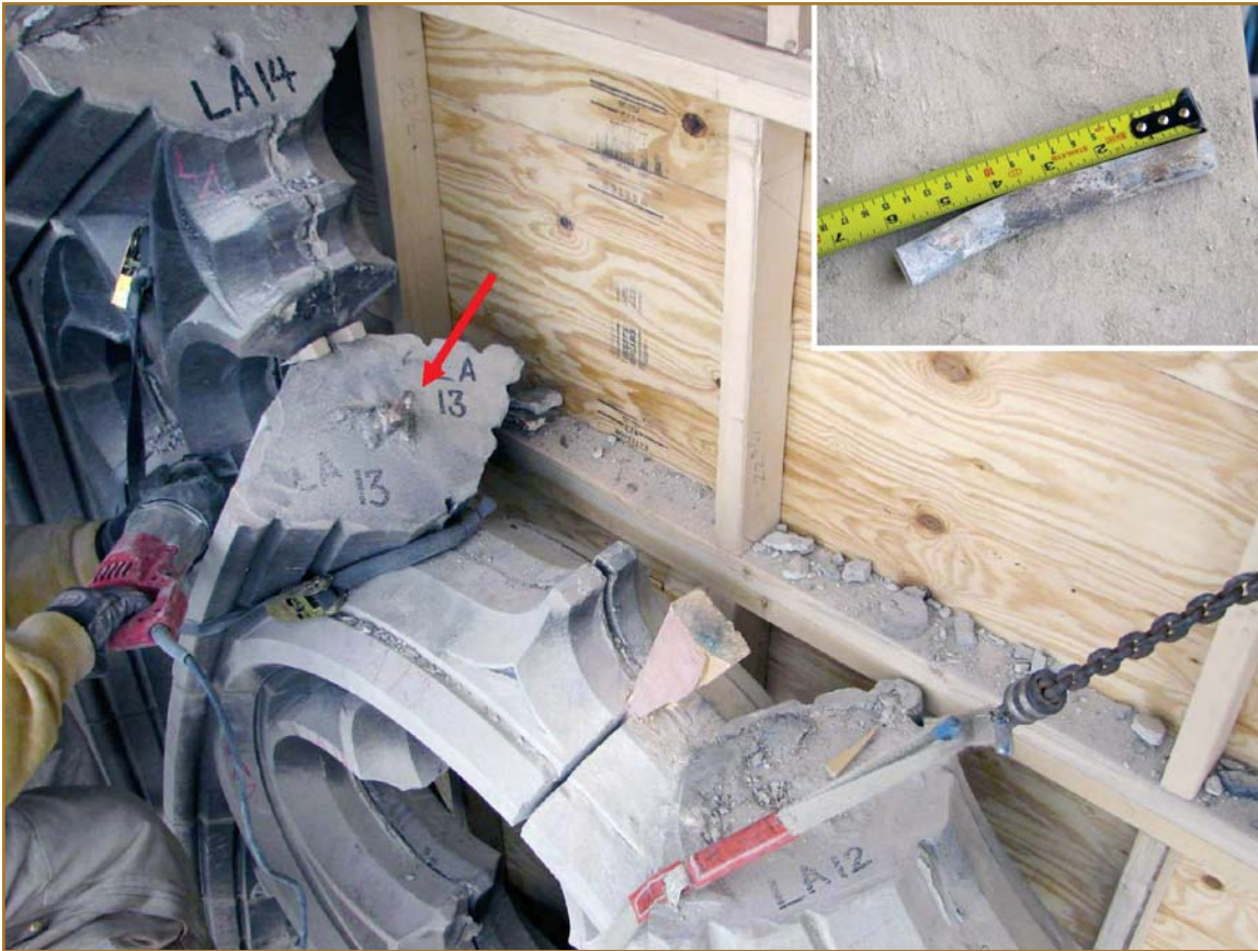
Photo 18 – Overall condition of steel pins at stone cusps from the organ loft window location.
