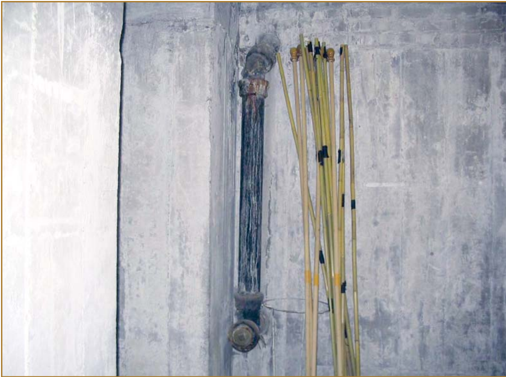
Figure 1, Condition C – Typical drain leader exiting the buttress as presented in the basement.
