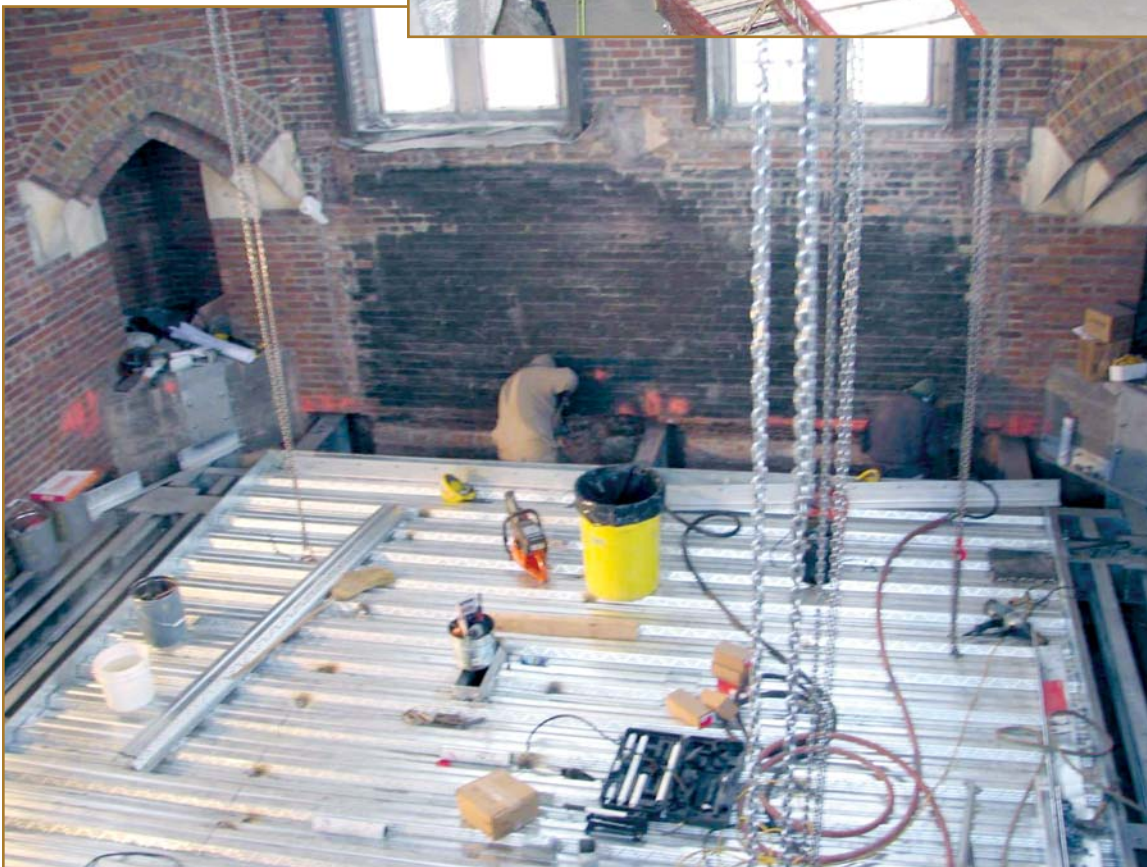
Photo 21 – Ironworkers set new steel framing and decking for the playing cabin at the 160-ft level of the tower interior.
