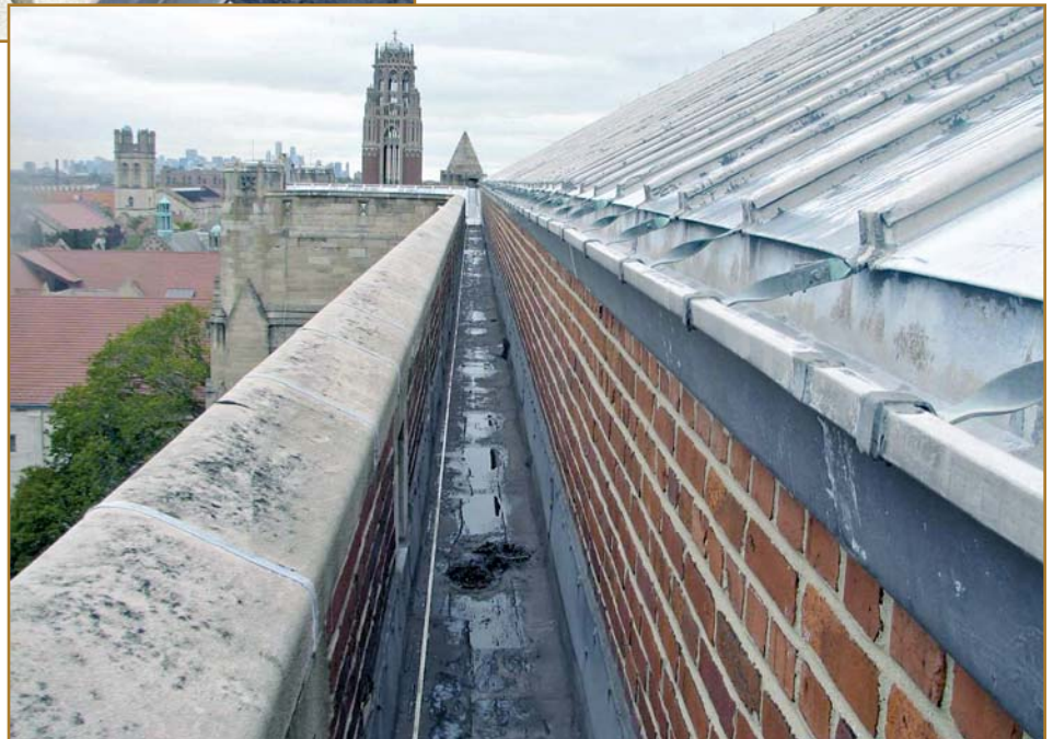
Photo 9 – Typical integral gallery at the east and west sides of the nave (below).
