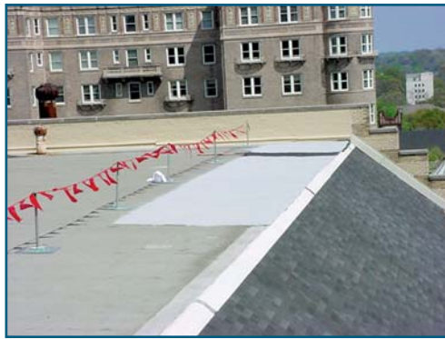
View of the mansard edge, which originally leaked due to differential movement from a buried I-beam at the perimeter.
