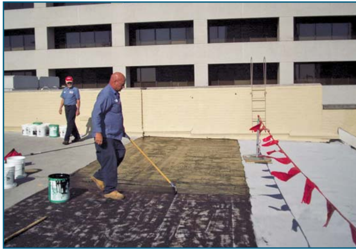
Application of cold-process surfacing adhesive over primed surface prior to granule application.
