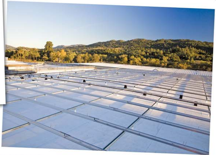
Completed roofs, standoffs, and solar racking system prior to panel installation at Asti Winery in Cloverdale, CA.
