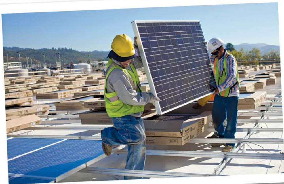
Solar panels are installed at Beringer Vineyards in St. Helena, CA.
