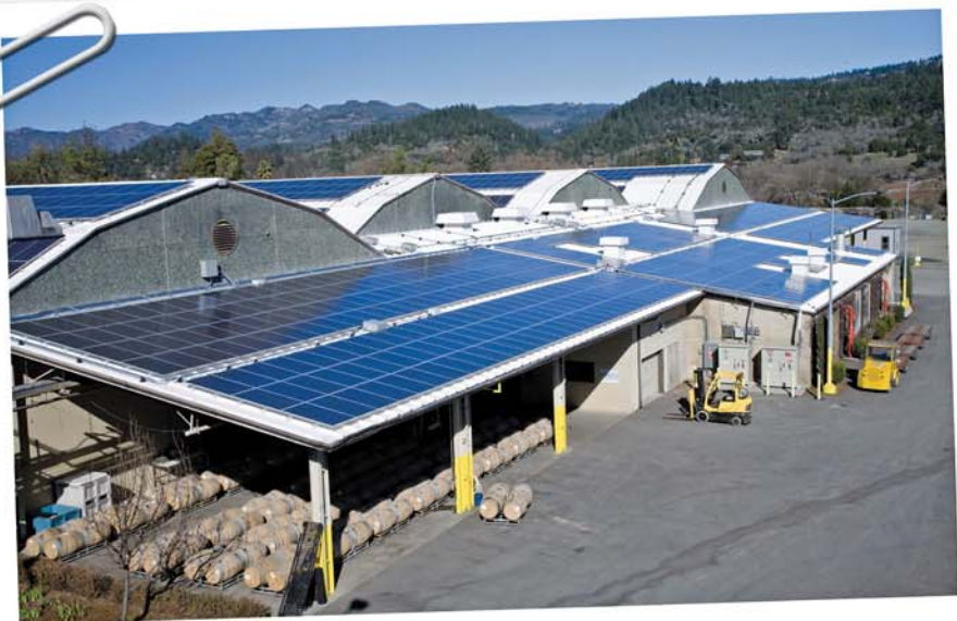
Roofline view of the solar installation at Beringer Vineyards in St. Helena, CA.
