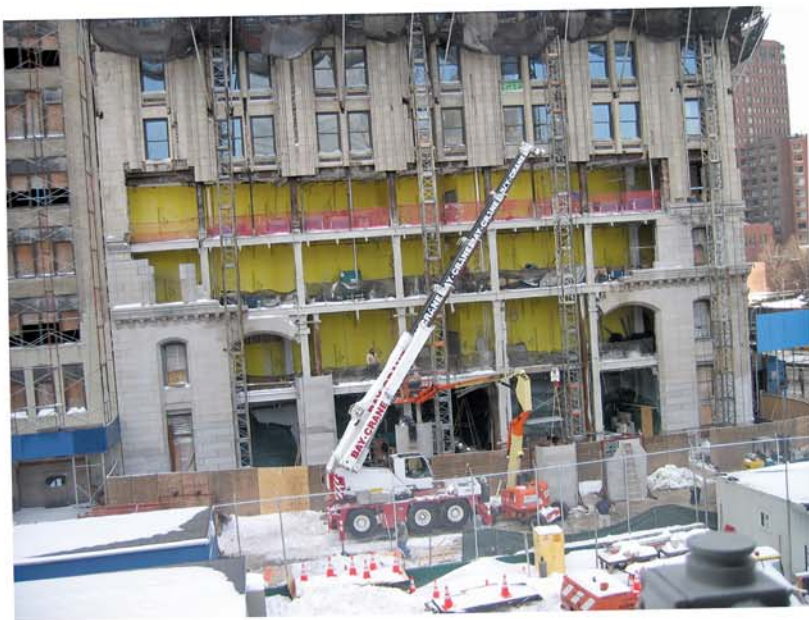
Figure 19 – Most of the north granite façade base was completely removed.
