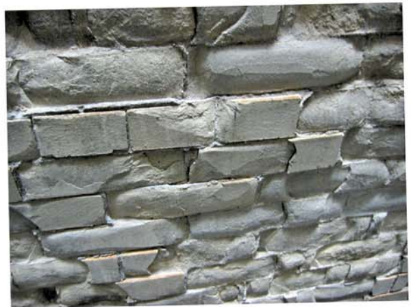
Figure 9D – Brick spalls due to heat of fire in the courtyard.
