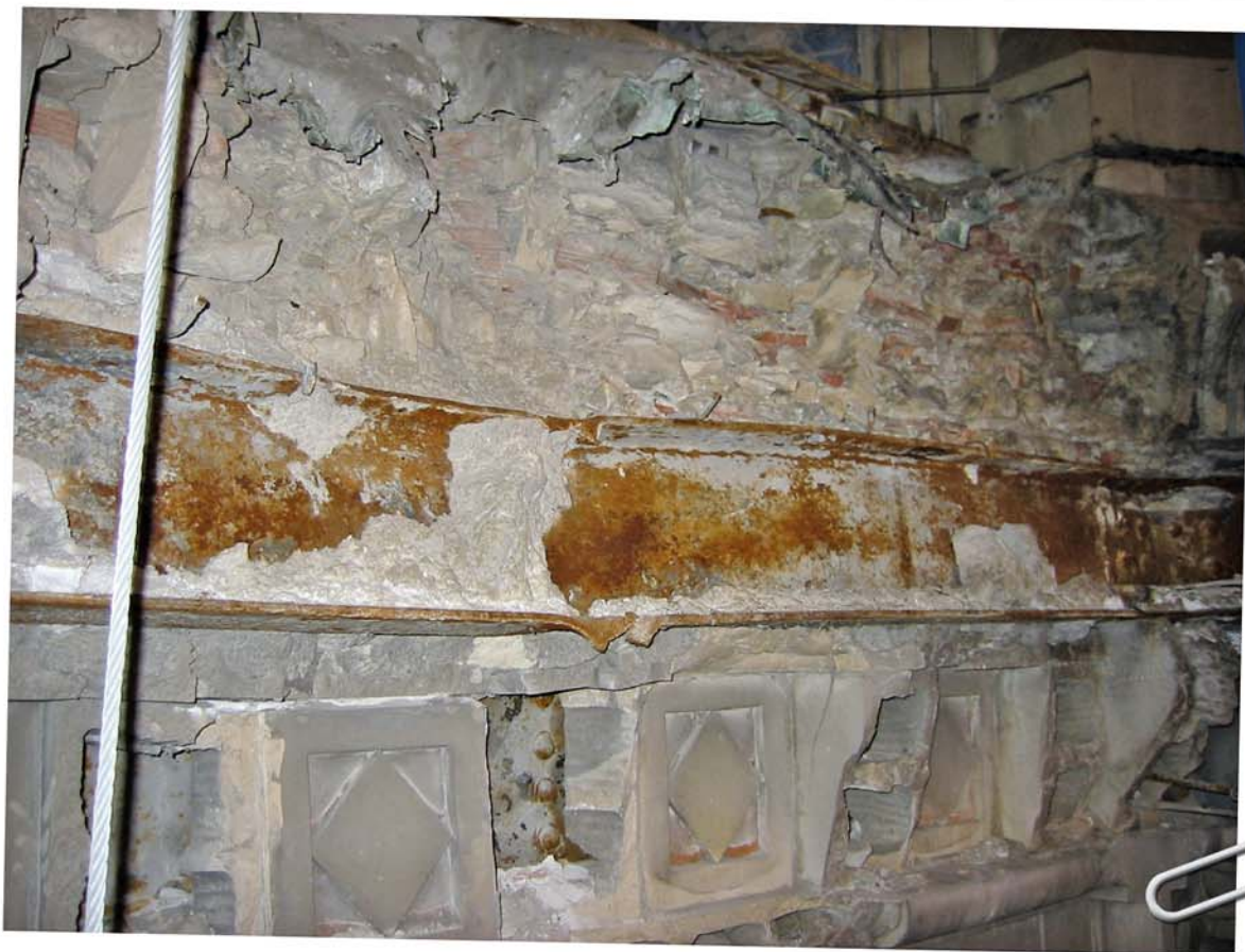
Figure 7 – North façade. Impact damage crushed terra cotta and bent and nearly sheared through a steel spandrel beam.
