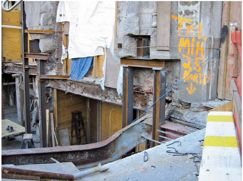
Figure 18 – Much of the north sidewalk, which supported the granite, was missing.
