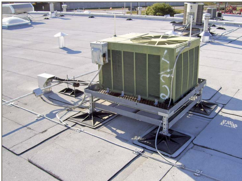
Figure 13 – Mechanical equipment installed on pre-manufactured support.
