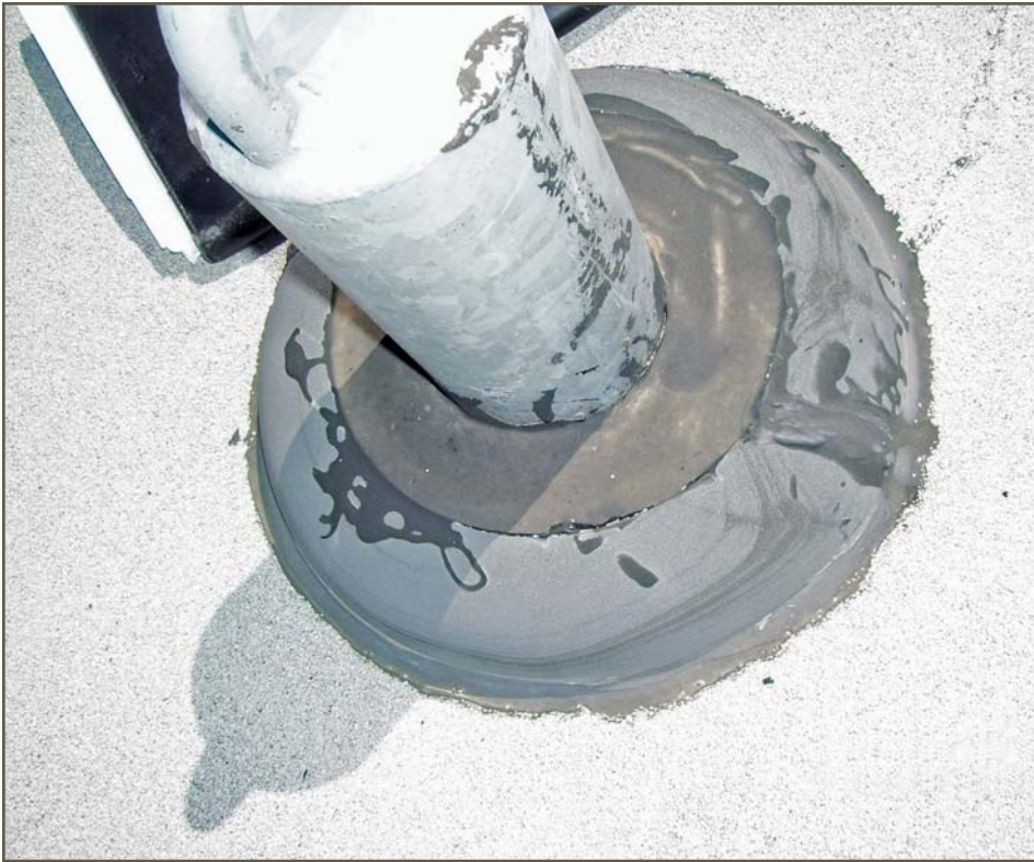
Figure 8 – Pre-manufactured penetration seal (“doughnut”) installed at steel support.
