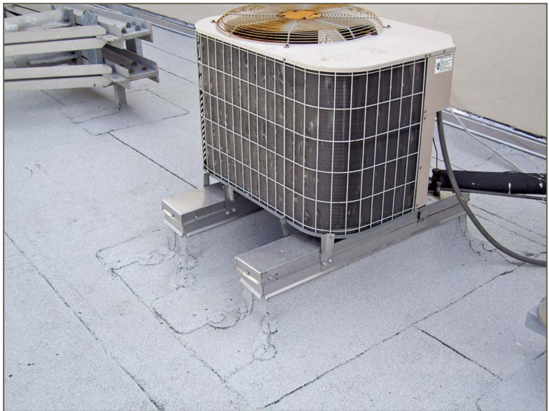
Figure 4 – Equipment installed on curbs/runners.
