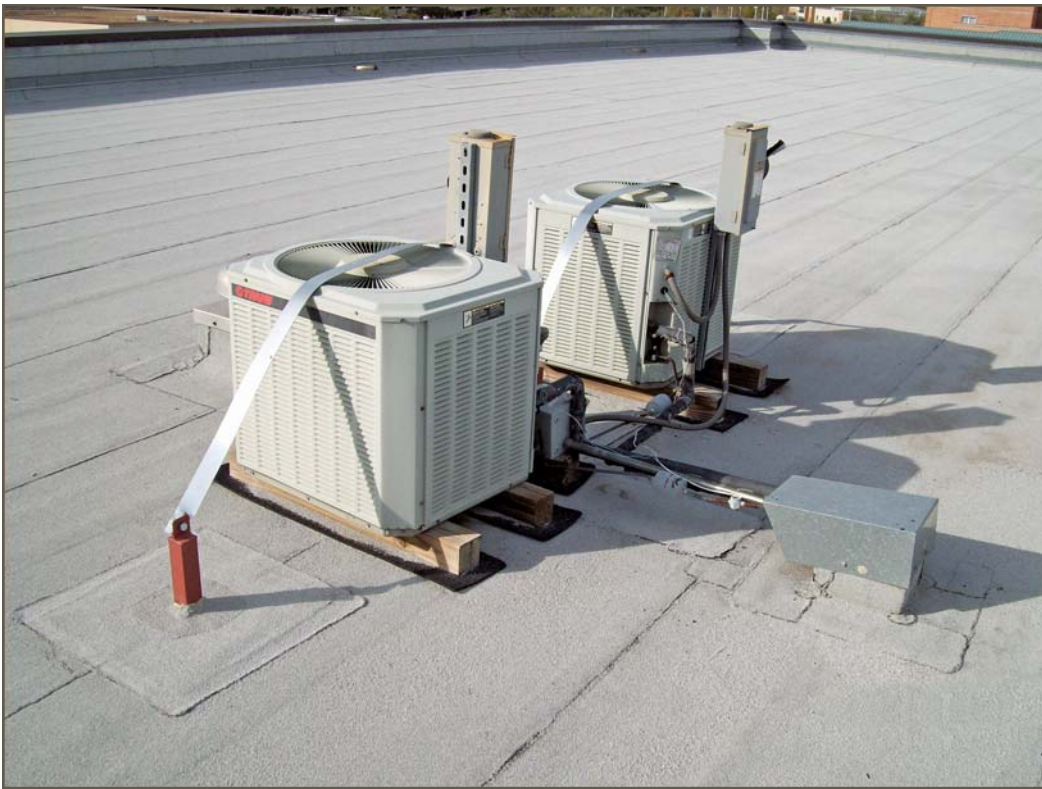
Figure 10 – Equipment installed on top of 4x4 wood sleeper.
