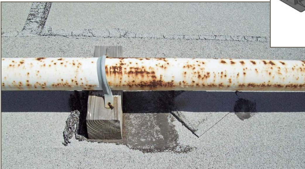
Figure 11 – Damage to roof from movement of piping and support.
