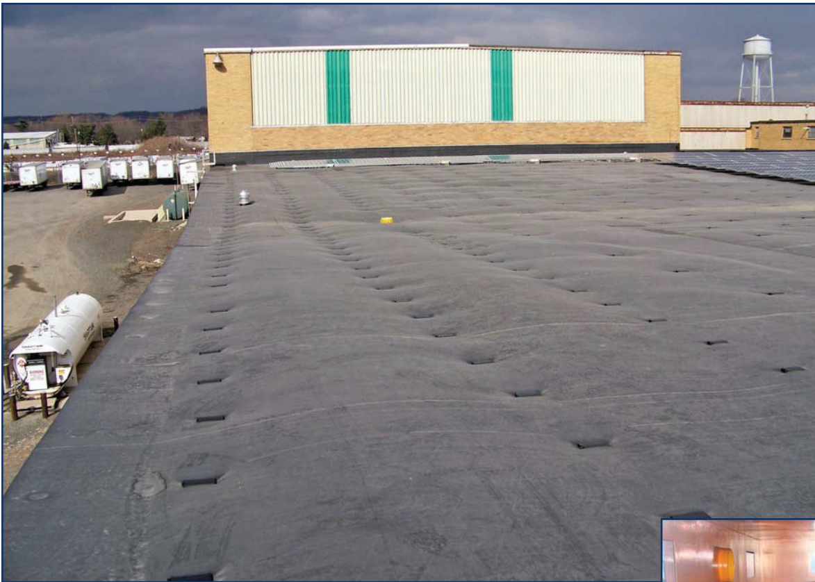
Figure 1C – Billowing of mechanically attached EPDM membrane in the field. (Photo, courtesy of Tom Kelly).
