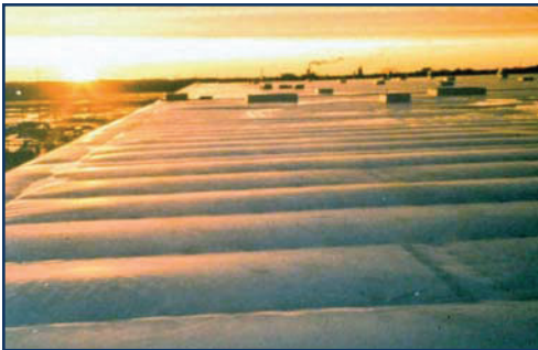
Figure 1A – Billowing of mechanically attached TPO membrane in the field (Photo courtesy of Hans Gerhardt).
