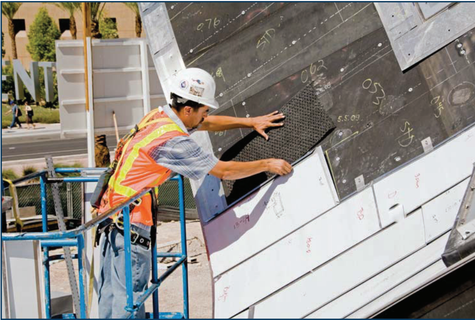
Figure 8 – Installation of an underlayment with incorporated structural separation layer under stainless steel panels at the Cleveland Clinic Lou Ruvo Center for Brain Health in Las Vegas, NV.
