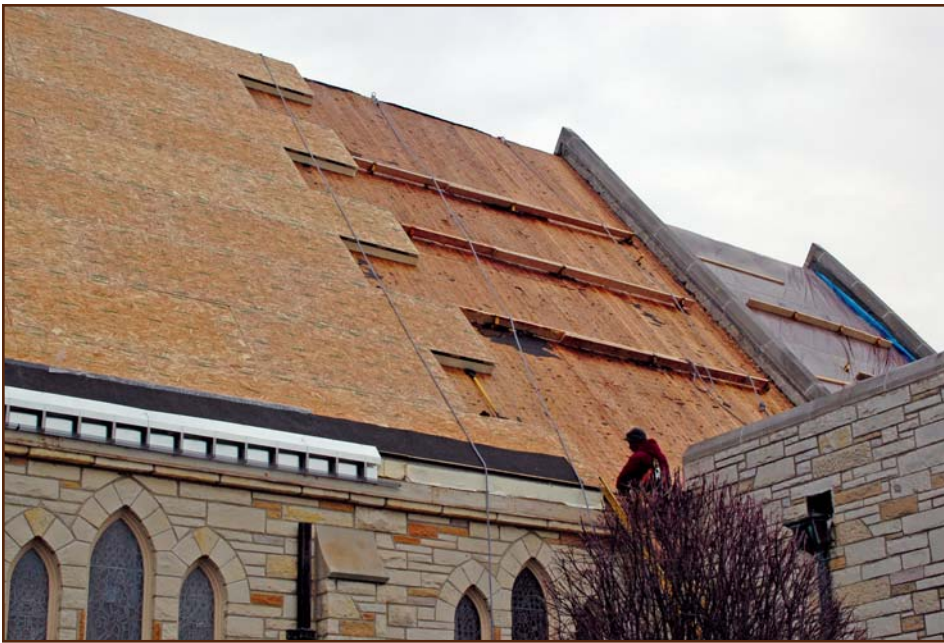
Figure 10 – A partial installation of the vented nail base on St. John’s Lutheran Church.
