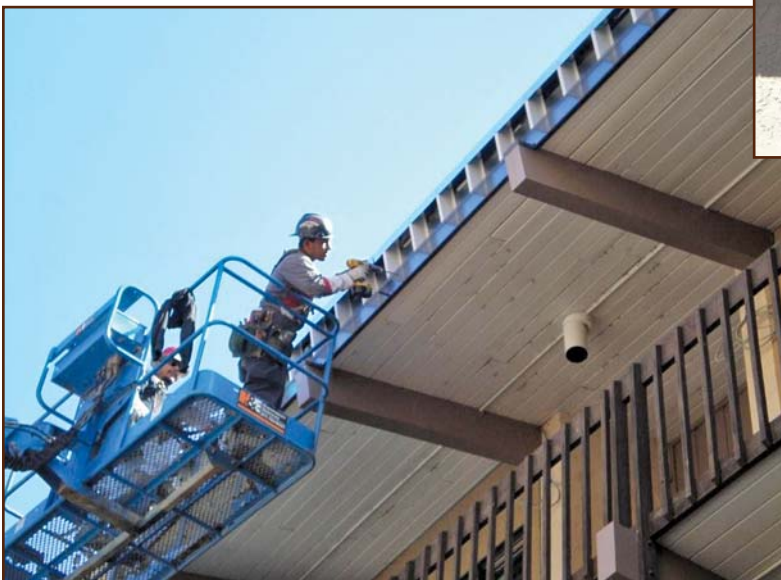
Figure 3 – A vented fascia with the appropriate NFA is installed at the eave.
