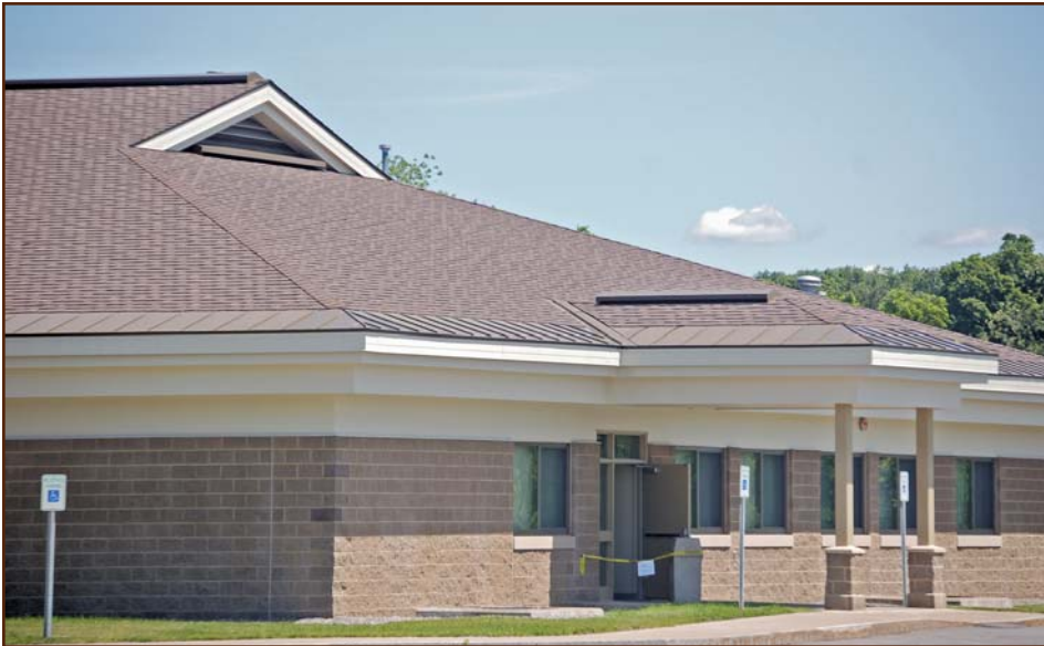
Figure 5 – Commercial ridge vents were installed on each roof level of the building.
