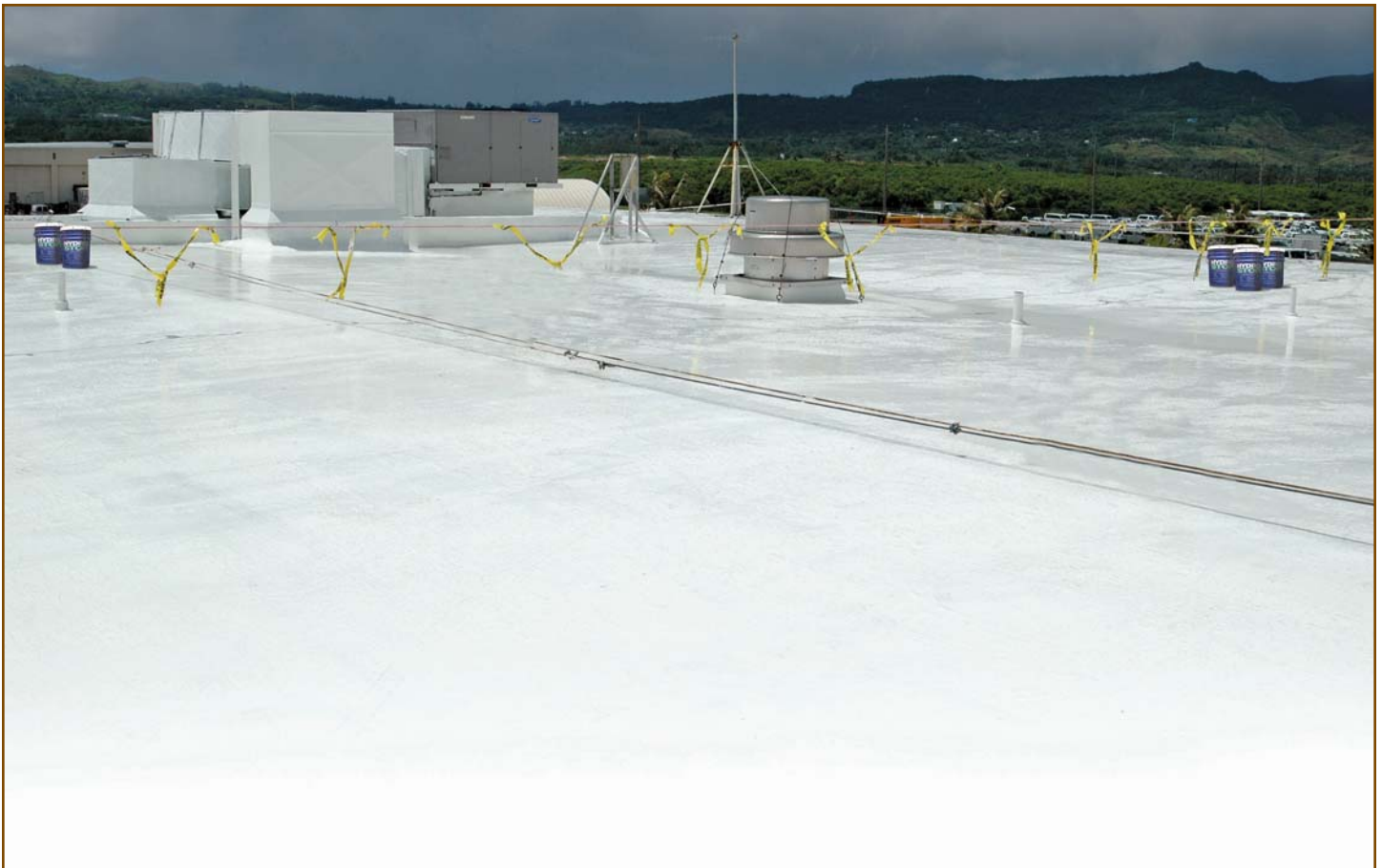
Photo 7 – A fast-setting acrylic coating was used on this building in Guam. (Photograph Courtesy of Quest Construction Products: United Coatings, Spokane, WA.)
