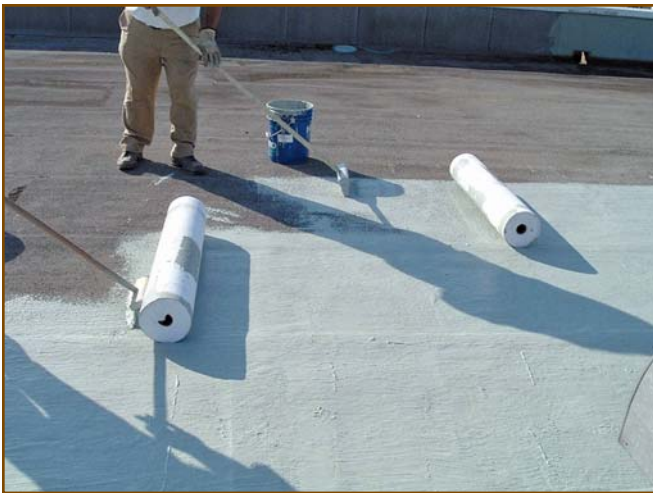
Photo 2 – Workmanship and extensive use of fabric bring new life to an old mod-bit roof, with a monolithic, adhesively attached acrylic membrane. (Photograph courtesy of Quest Construction Products: United Coatings, Spokane, WA.)
