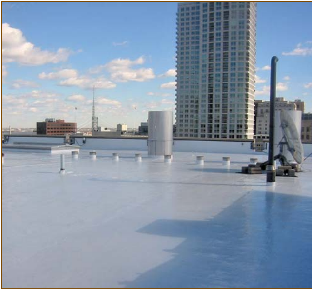
Photo 6 – Silvery-metallic, aluminum-asphalt coatings are economically important because of their proven effectiveness in extending roof service life. (Photograph courtesy of the Garland Company, Cleveland, OH.)
