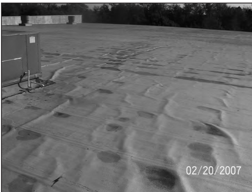
Figure 6 – Example of wind uplift damage to a portion of a smooth-surfaced modified-bitumen roof membrane.
