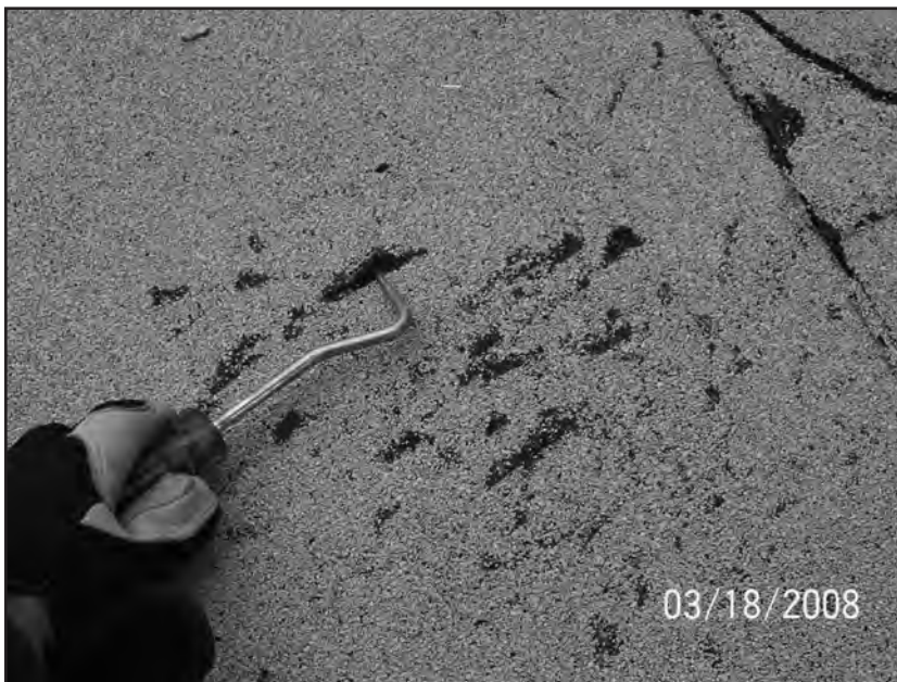
Figure 5 – Example of storm damage to granule-surfaced modified-bitumen membrane from glass debris.
