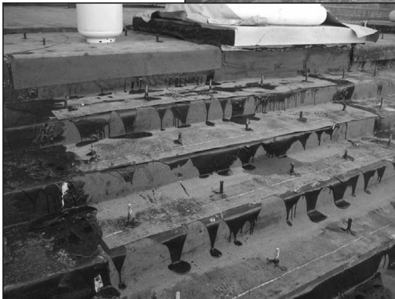
Photo 17 – Protection board cut into smaller and more manageable pieces that lap several inches onto each tread near the nose of the stair, over the vertical riser, and over the majority of the tread below the riser. Note that the protection board conforms to the shape of the stairs.
