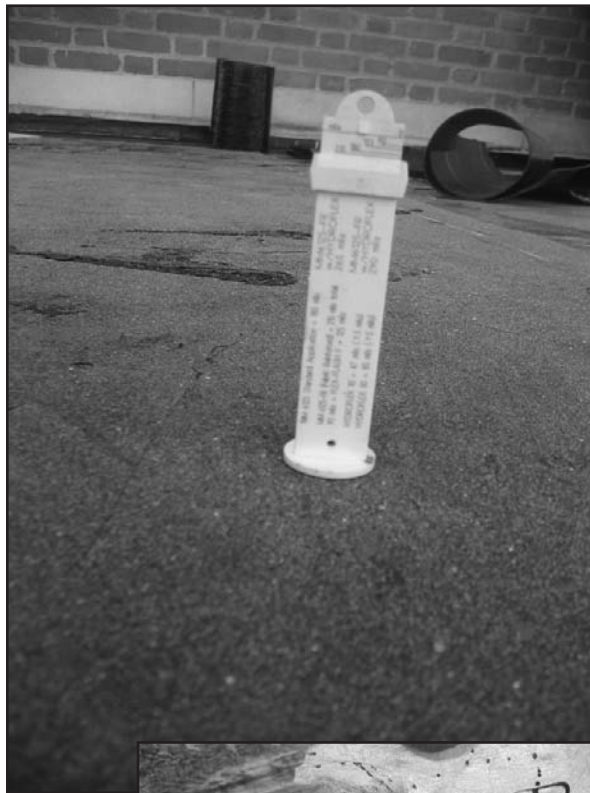
Photo 9 – Measurement of membrane thickness with pin tester. Note that the pin (not shown) is inserted into membrane and thickness is read off the top (arrow).
