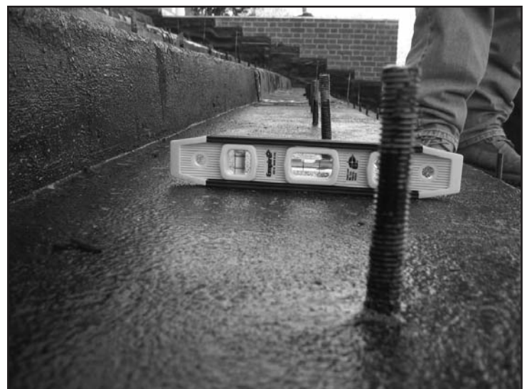
Photo 3 – Level showing sloped surface at a stair tread. We added slope with a concrete topping at the stair treads to promote drainage.
