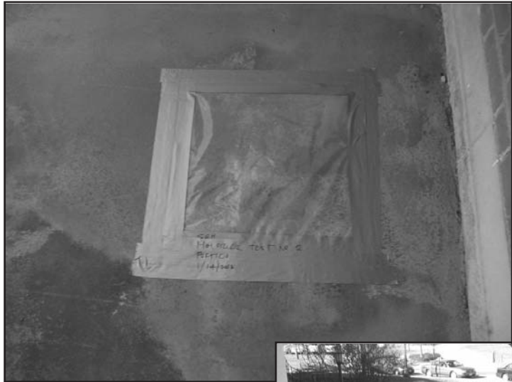
Photo 4 – Moisture test according to ASTM D 4263 – Standard Test Method for Indicating Moisture in Concrete by the Plastic Sheet Method.
