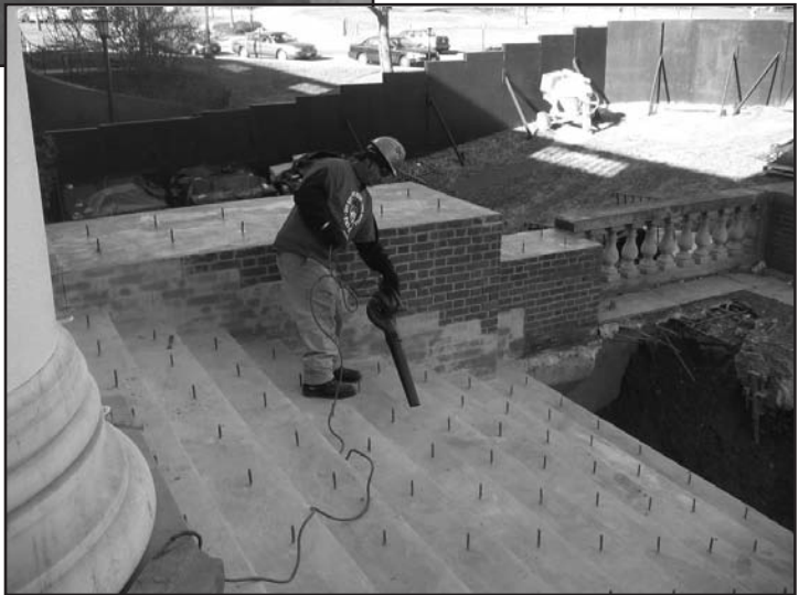
Photo 5 – Removal of dirt and debris from concrete surface using a hand-held blower.
