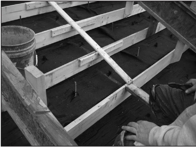
Photo 18 – Continuous layer of drainage board that conforms to the shape of the stairs.
