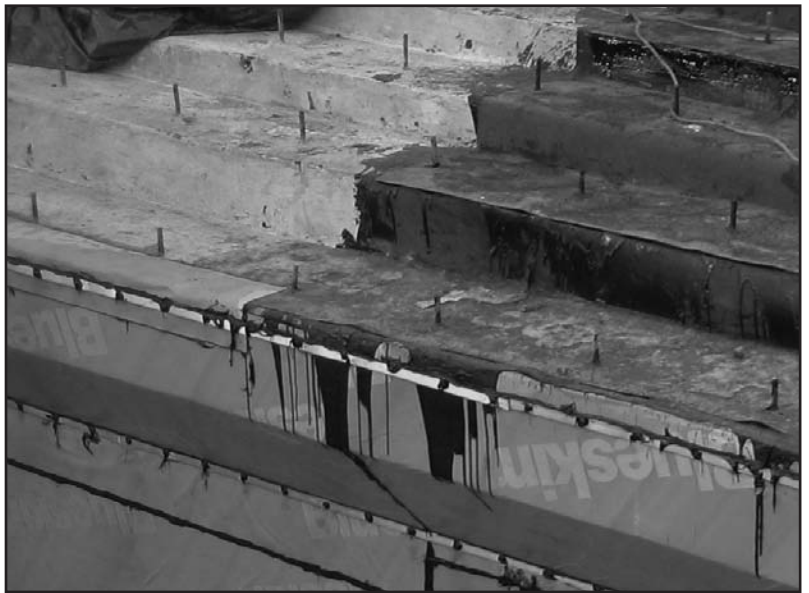
Photo 12 (above) – Hot-fluid-applied, asphalt waterproofing membrane lapped over self-adhered waterproofing membrane at the vertical foundation wall.
