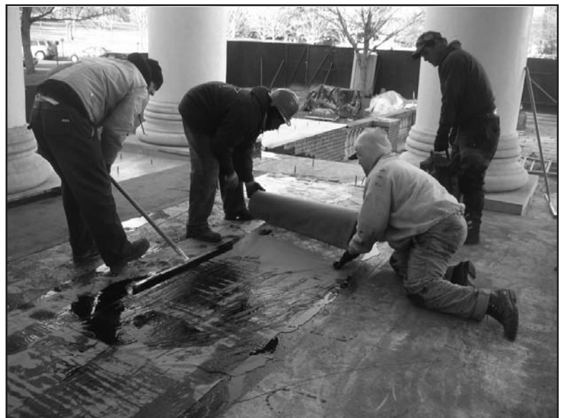
Photo 8 – Placement of fabric reinforcement on top of the first coat of membrane.
