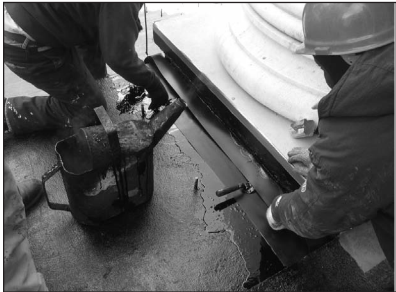
Photo 11 – Neoprene flashings installed at the base of a portico column prior to the application of waterproofing membrane.
