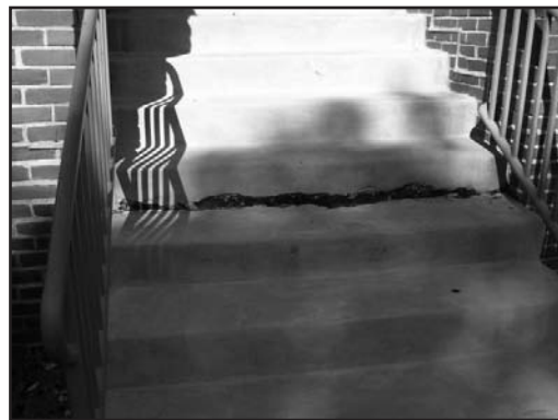
Photo 19 – Stain at stairs installed over hot-fluid-applied, rubberized asphalt waterproofing with no drainage layer at a waterproofing project.
