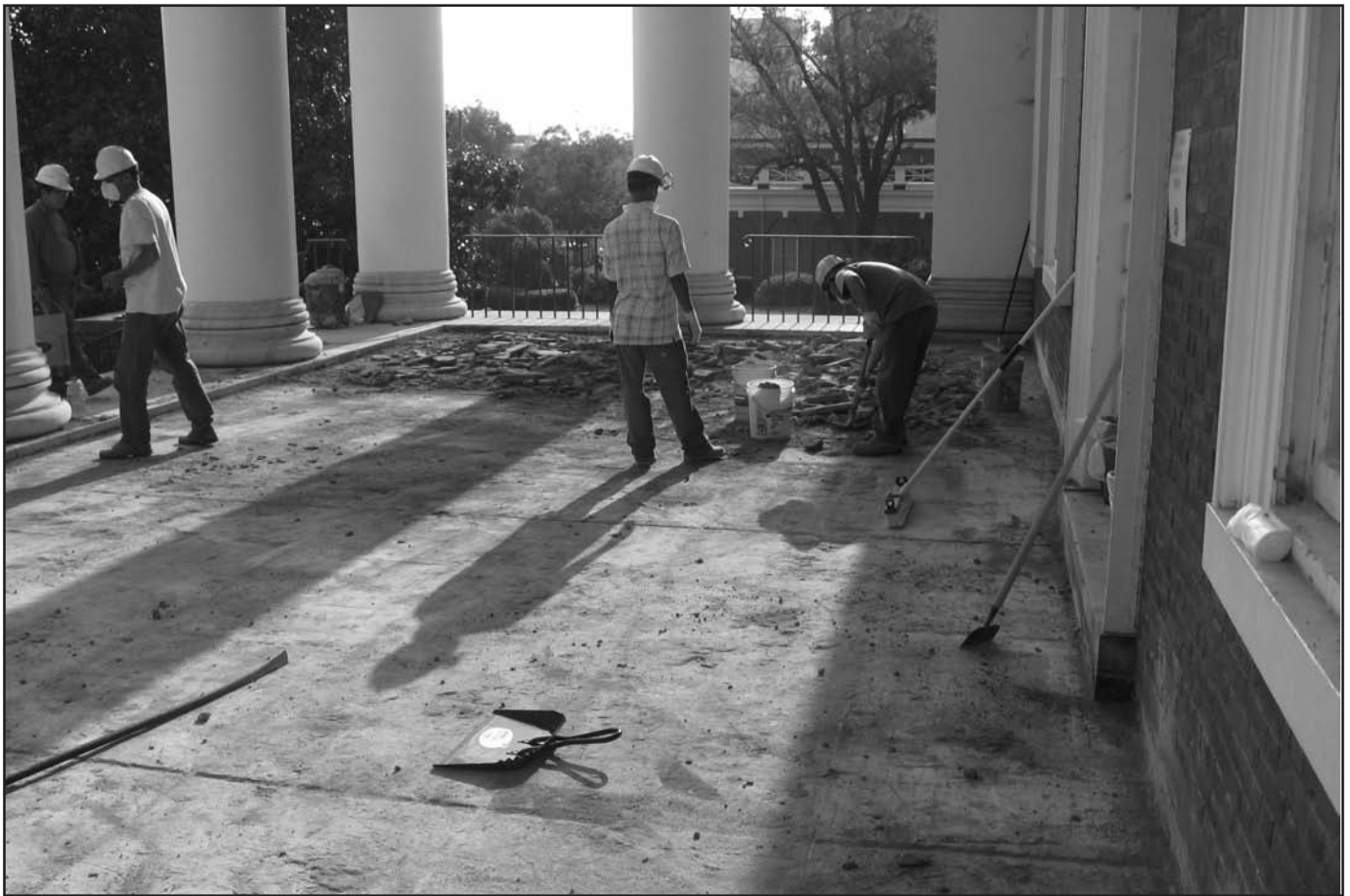
Photo 1 – Removal of concrete topping over concrete substrate. Note the existing roofing system consisted of (from interior to exterior): concrete deck, existing waterproofing membrane, concrete topping slab, mortar setting bed, and overburden (not shown).
