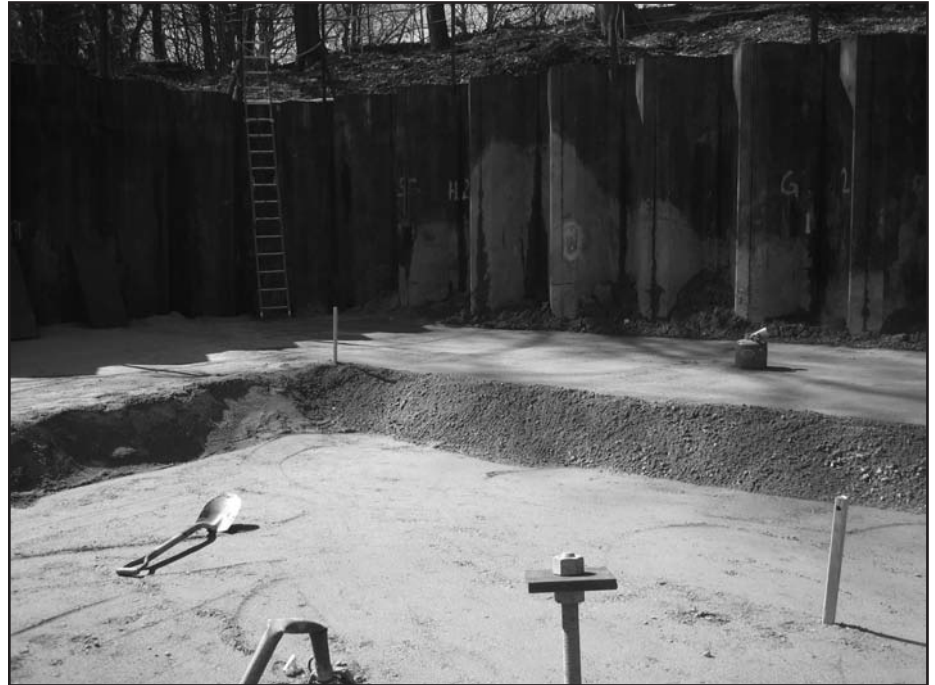
Photo 1 – View of compacted, engineered backfill material prior to application of waterproofing and pouring of the concrete foundation slab in a blindside application.
