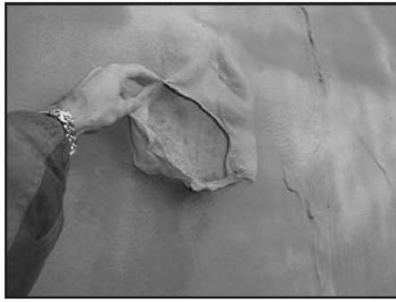
Photo 6 – Blister in a fluid applied waterproofing application.
