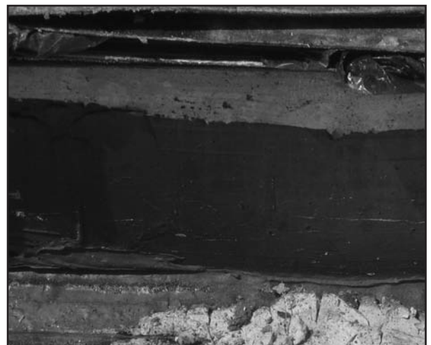
Photo 3 – View of unconfined and prematurely hydrated bentonite waterproofing. Bentonite waterproofing can swell up to 15 times its dry volume.
