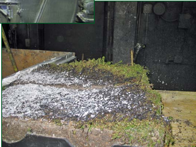
Photo 11 – No damage to anything other than the top cover exposed to direct flame. (Photo courtesy of DLR Consultants.)
