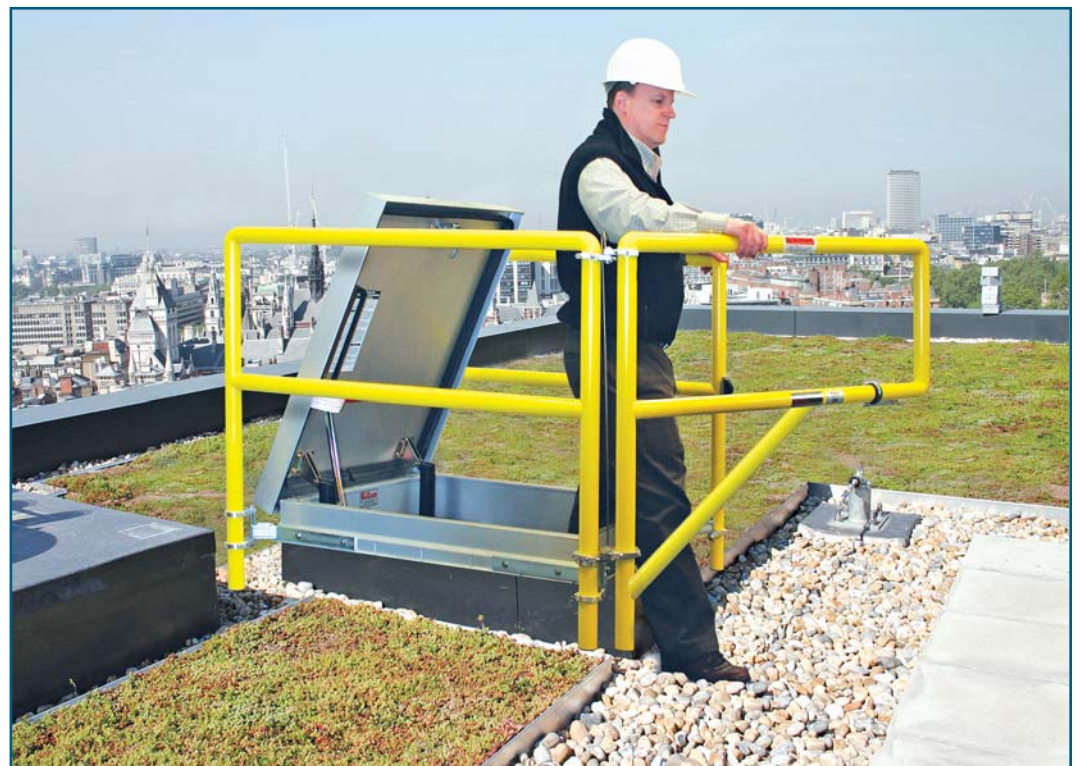
Photo 3 – This ladder-access hatch has a hatch railing system, which satisfies OSHA 29 CFR 1910.23 standard by ensuring continuous fall protection around the hatch opening.
