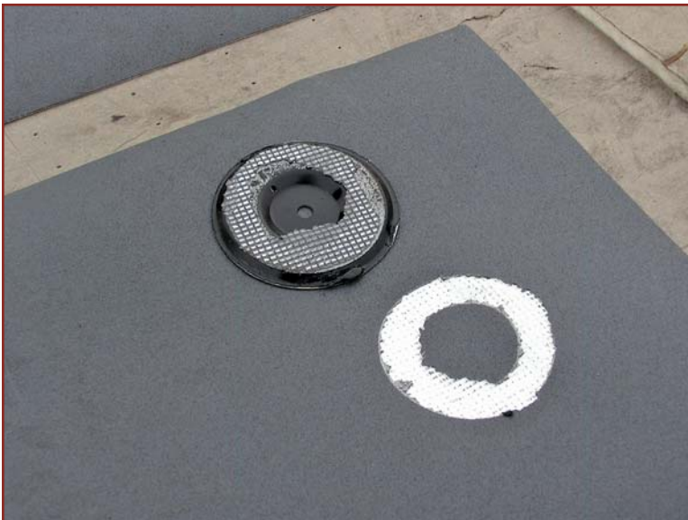
Photo 6 – The tool must be calibrated based on the ambient temperature to provide an optimal bond. A properly bonded plate will provide total, even, and consistent fusion of the membrane.
