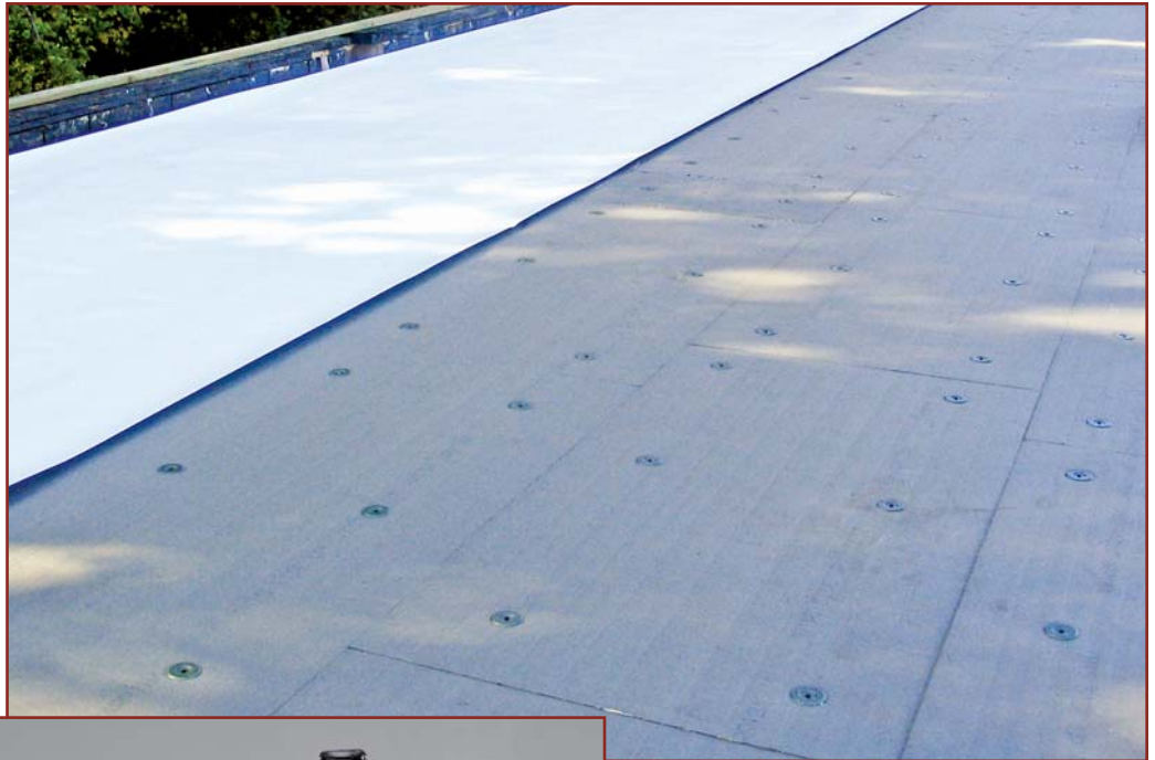
Photo 4 – Fasteners are installed across the entire roof in a grid pattern to distribute the wind load more evenly. Membrane width is inconsequential, with no need for perimeter half sheets.
