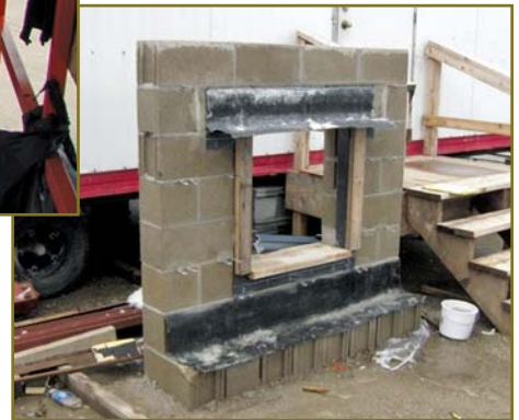
Figure 6 – Window-wall “mock-up” that was quite different from the designer’s intent.
