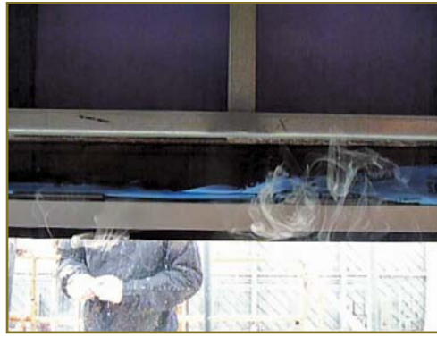
Figure 9 – Qualitative airtightness smoke test showing concentration of air leakage over small area on a mock-up where quantitative airtightness-test results indicated a “pass.”
