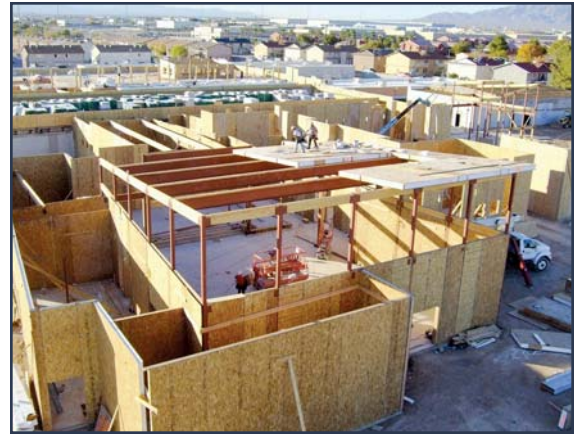
Figure 5 – SIPs were used on the 68,000-sq-ft Jacob E. Manch Elementary School in Las Vegas, Nevada. With 500 skylights installed in the SIP roof, the school uses 100% daylighting.
