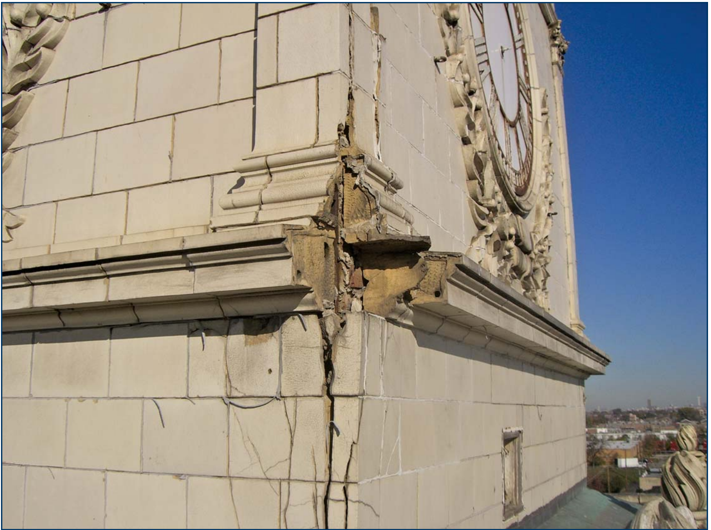
Figure 3 – Distress of masonry cladding resulting from corrosion of embedded steel structure.
