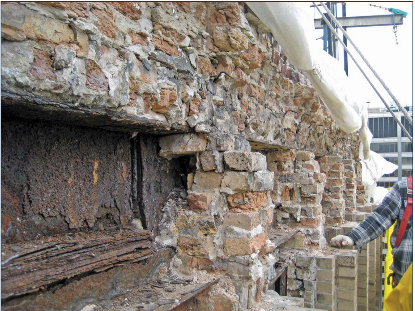
Figure 6 – Corroded steel revealed following removal of terra cotta cladding.
