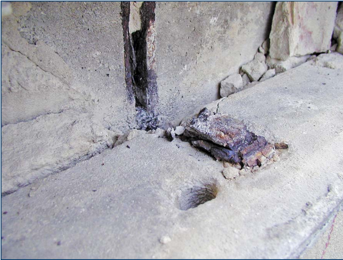
Figure 8 – Complete loss of lateral anchorage.
