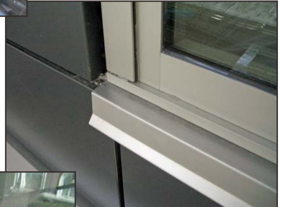
11: Type III – SAF pan – concealed for block-frame window in metal panel cladding. Aluminum sill cover protection over pan flashing.
