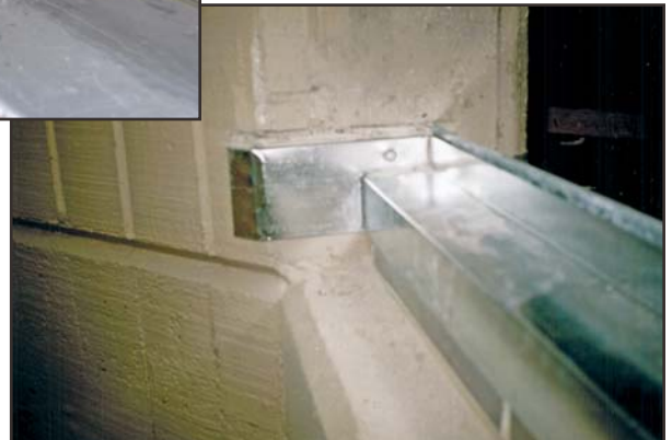
6: Type I – GSM pan – direct drain for block-frame window in concrete opening.
