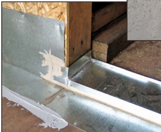
5: Type I – GSM pan – concealed, for block-frame door in flush stucco opening and elastomeric deck.
