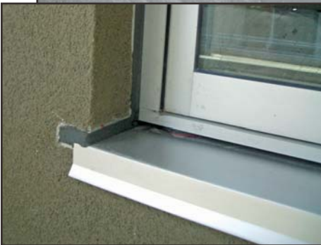
13: Type III – SAF pan – concealed, for block-frame window in recessed stucco opening. Aluminum sill cover protection.
