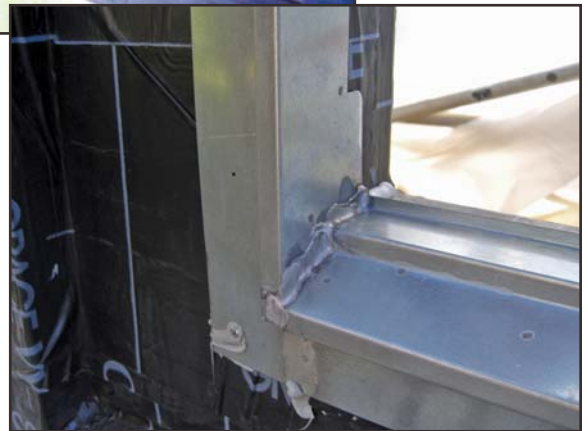
2: Type I – GSM pan – direct drain for block-frame window in recessed stucco opening.
