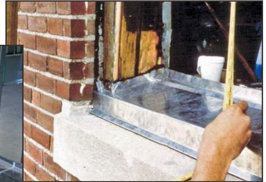
9: Type III – GSM pan – direct drain for block-frame window in masonry opening.
