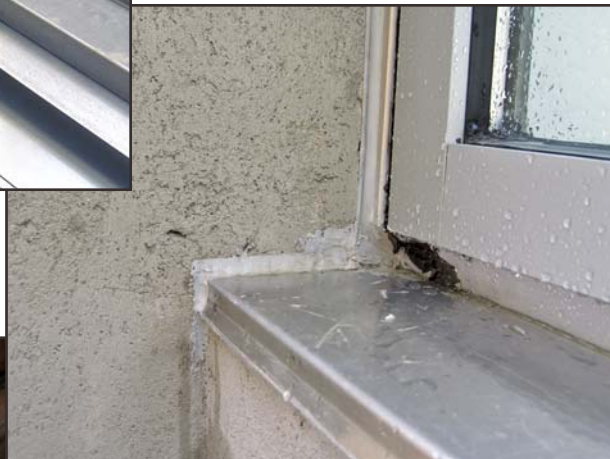
4: Type I – Aluminum pan and sill cover – direct drain for block-frame window in recessed stucco opening.
