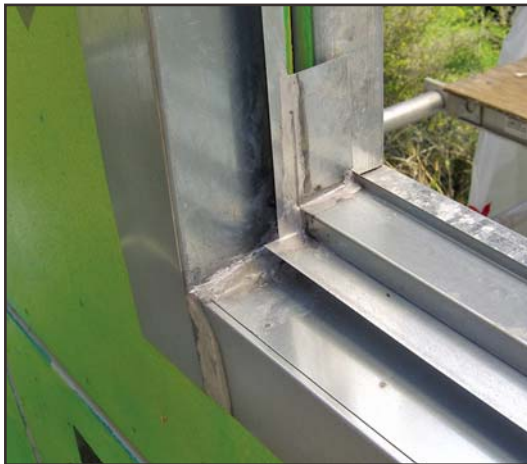
(Left) 3: Type I – GSM pan – concealed, for block-frame window in recessed stucco opening.
