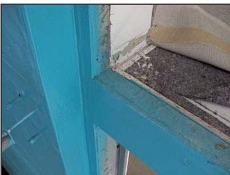
14: Type V – Liquid-applied sill protection to flush opening. A Type I – multiple pieces pan will go over the sill.
