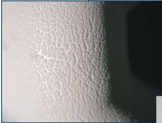
Photo 7 – PVC membrane #3 (14,000 hours).
