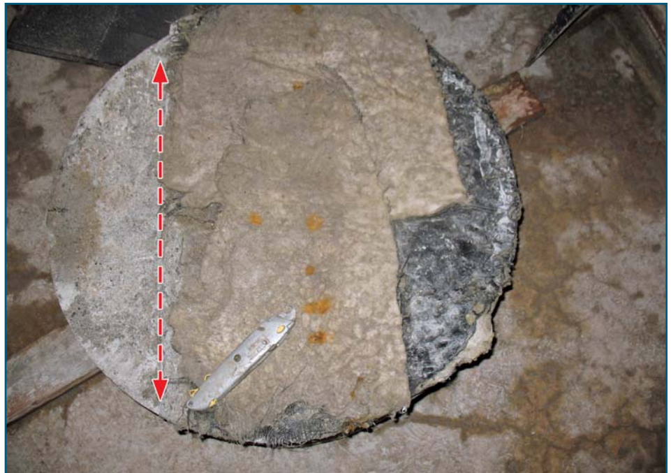
Figure 5 – Membrane layers on underside of core. Section on footing to left of dotted line.
