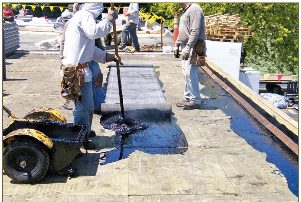
Photo 7 – Modified bitumen is installed directly on the stone-wool insulation in hot asphalt.
