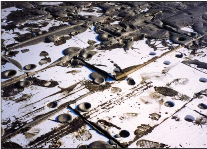
Figures 1 and 2 — What may first appear to be a random mess is instead a quite viable roof deck system. Here, polystyrene boards are situated into wet LWIC. The polystyrene provides the bulk of the R-value, while holes and slots in the boards provide a “keying-in” of these materials.
