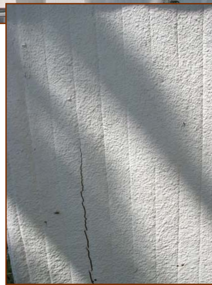
Figure 15 – Only damage after two hurricanes and 30 years of service.
