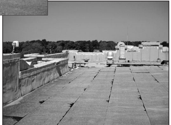
Photo 2 – Overview of existing roof systems. Note vertical wall flashings at back side of parapet.
