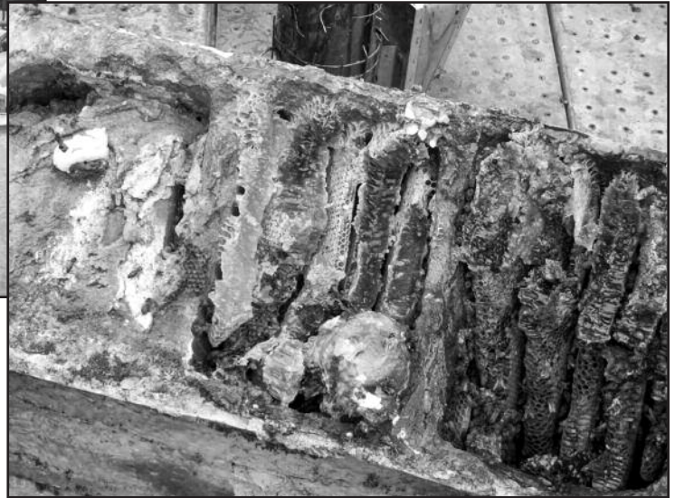
Photo 19 – Terra cotta void filled with honeycomb.
