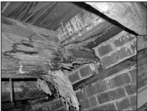
Photo 5 – Rotted wood rafter at bearing end, note box out for gutter.
