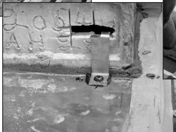
Photo 11 – Stainless-steel cleat at terra-cotta attachment.
