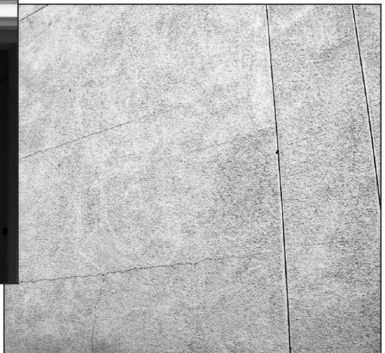
Photo 8 – Repetitive cracking patterns may conceal conditions requiring further investigation.
