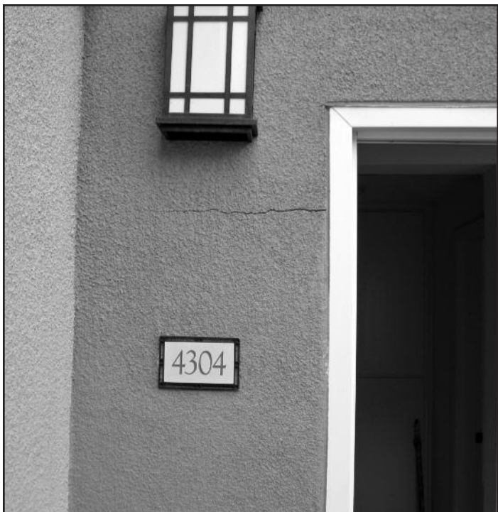
Photo 7 – Crack at entry door.
