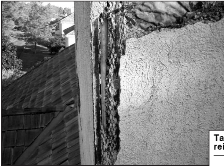
Photo 4 – Corroded metal lath.
