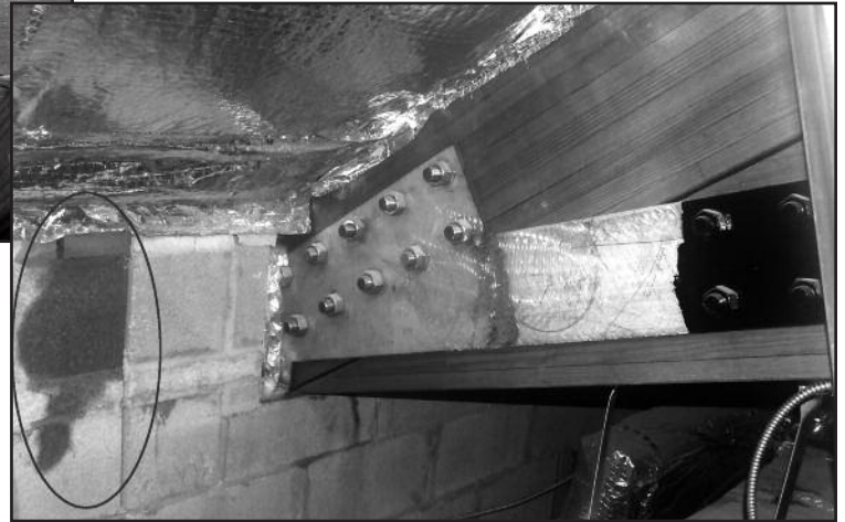
Figure 14 – View of condensation dripping from behind the FSK facing. It is not practical to tape FSK to CMU.
