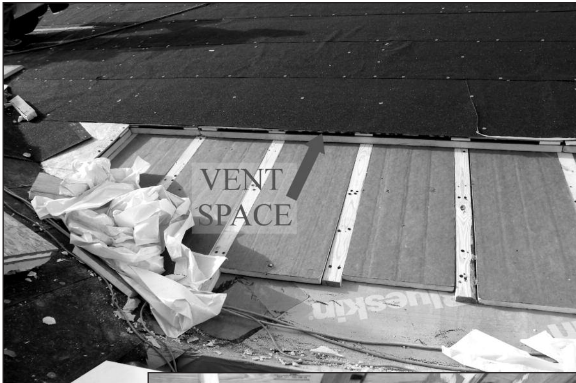
Figure 19 – View of the new 40-mil air/vapor barrier (blue), plus two layers of staggered polyisocyanurate rigid insulation, plus venting spacers, roof sheathing, and shingle underlayment.
