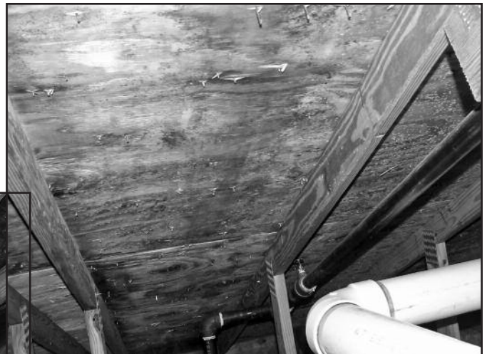
Figure 12 – Biological growth and buckled sheathing at the attic space above the aquatics office.
