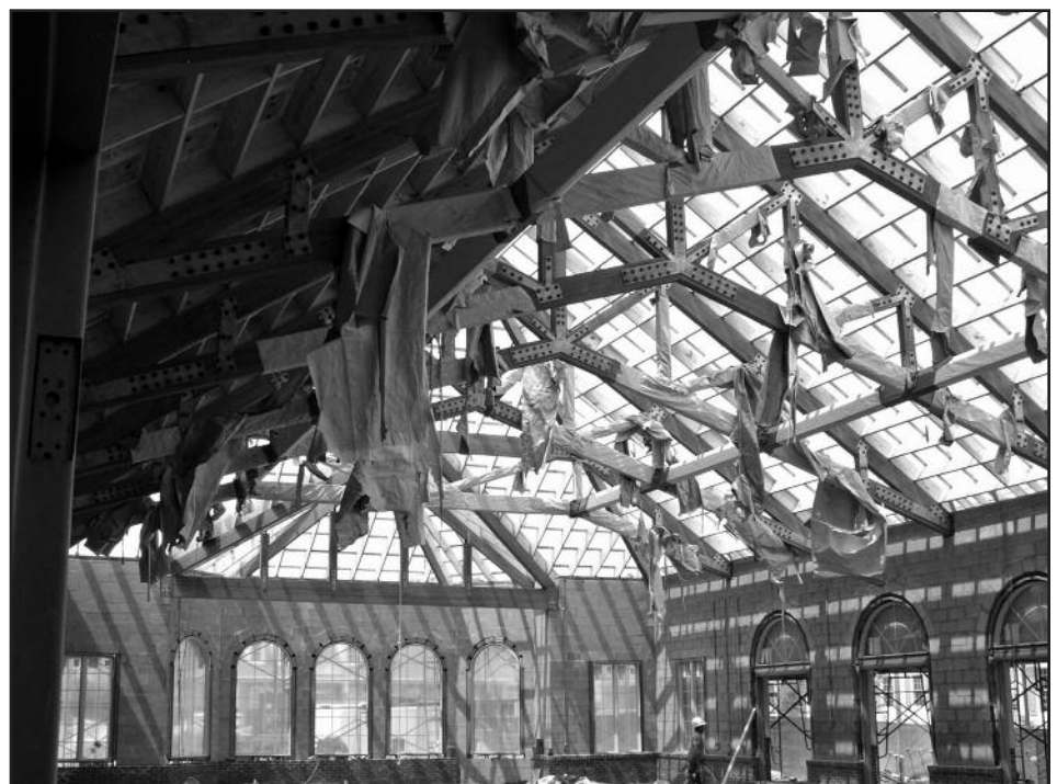
Figure 3 – View of original pool building roof structure under construction with truss protection wrap partially removed.
