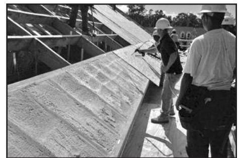
Figure 18 – View of SPF foam seal created at the building perimeter at the intersection of the top of the masonry wall and the roof eave. New sheathing supports 40-mil vapor barrier plus a ventilated roof assembly (not installed). Perimeter sheathing is set in wet foam and nailed to promote an airtight seal.
