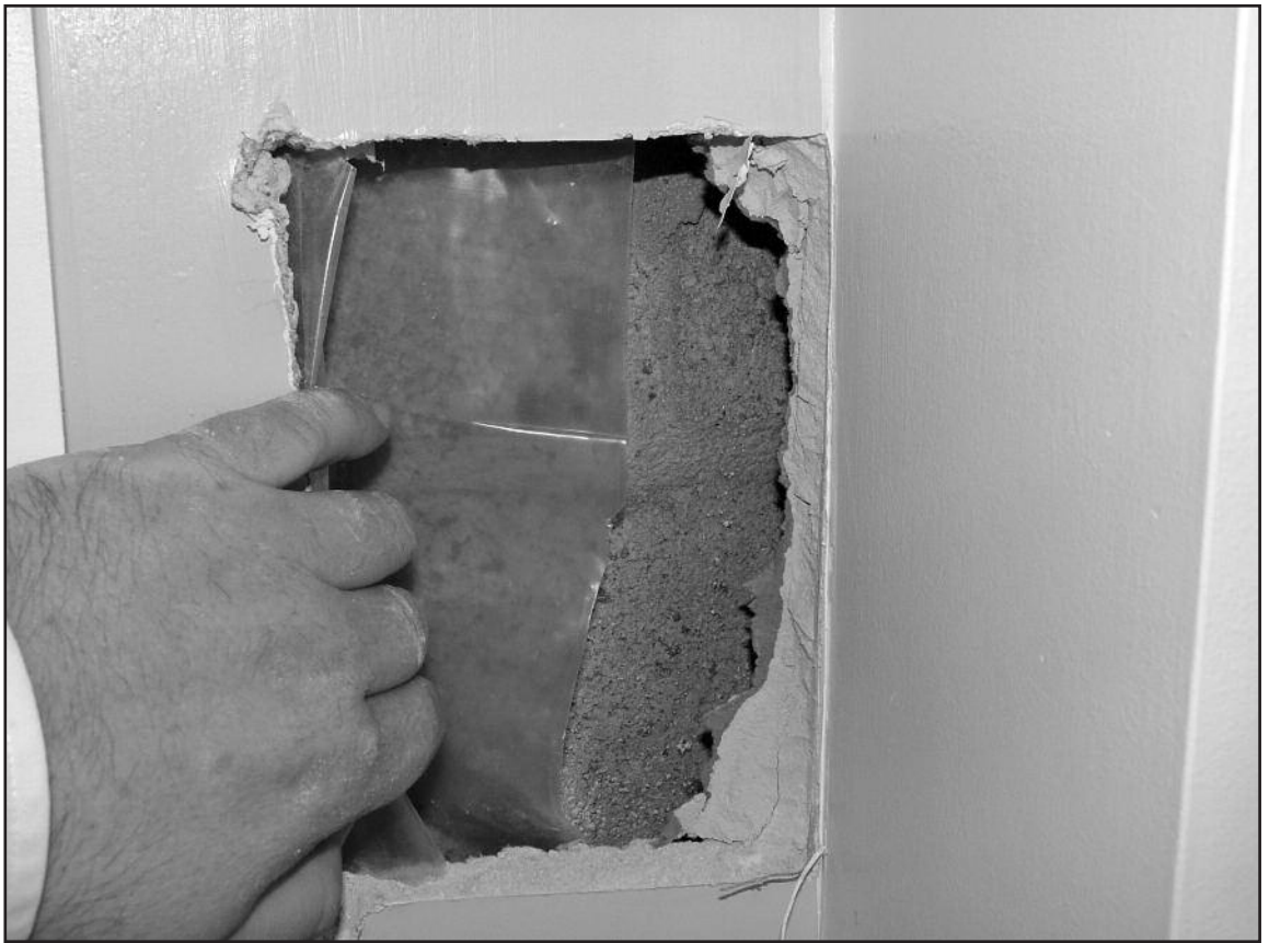
Figure 9 – In the walls, the polyethylene vapor barrier was not taped and sealed at all joints and laps.
