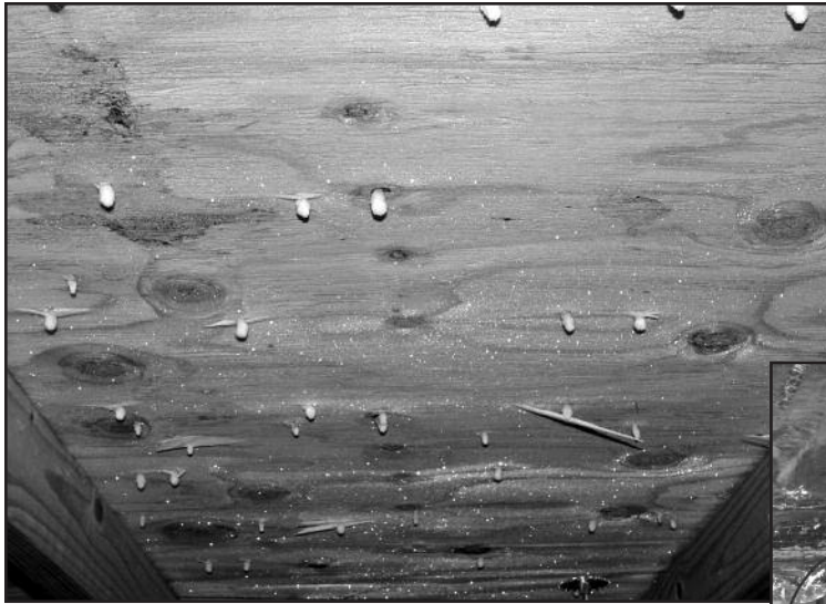
Figure 13 – View of condensation ice formation on the underside of the locker room attic roof sheathing.
