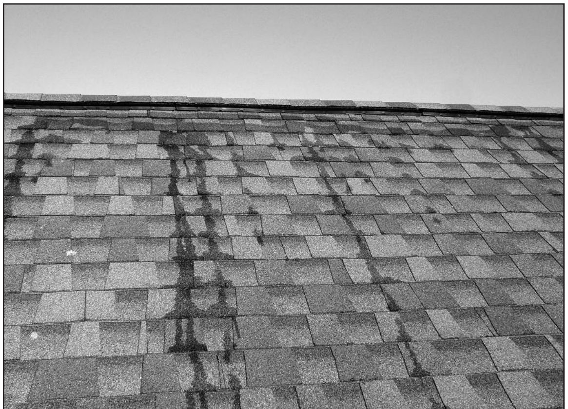
Figure 15 – View of condensation dripping from roof ridge vent.
