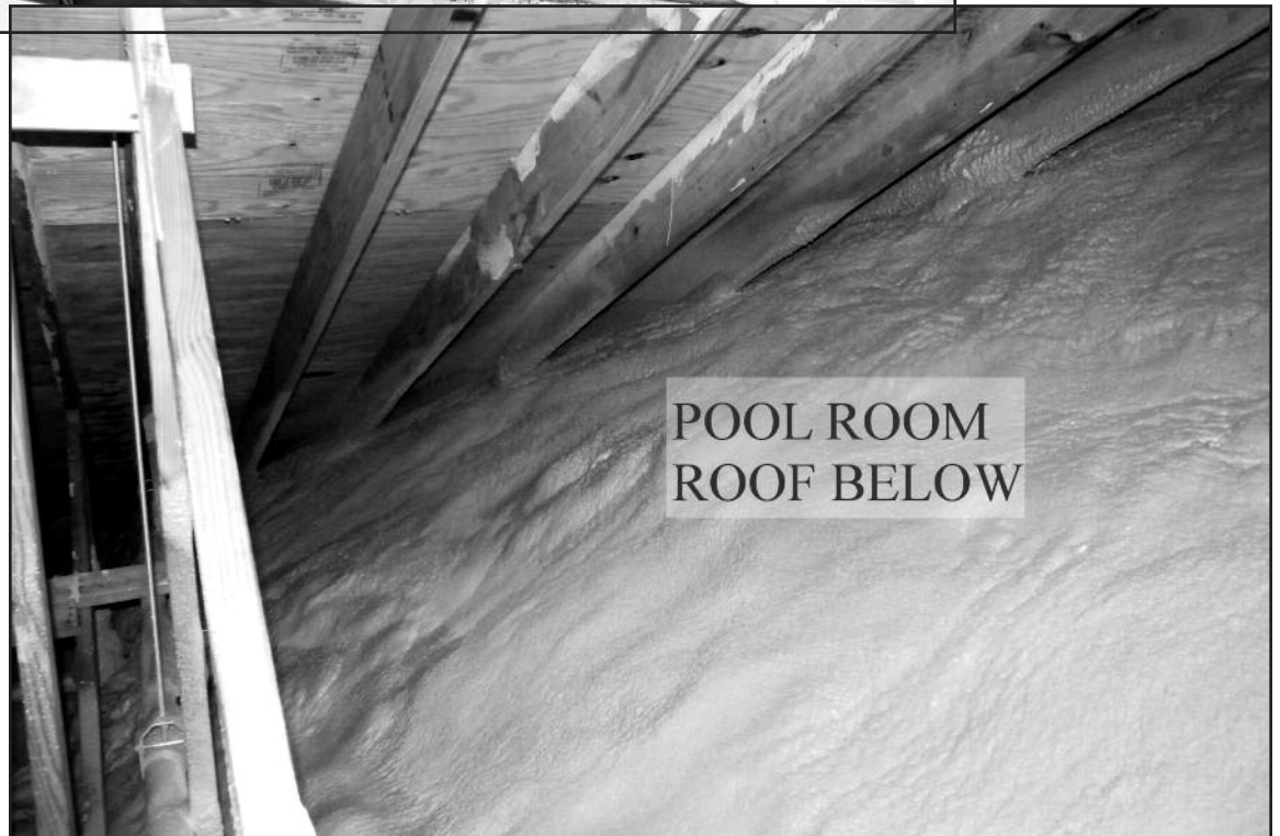
Figure 20 – View of SPF insulation installed in the adjacent attic creating an air/vapor barrier between the attic and pool-roof assembly prior to the application of an ignition barrier.
