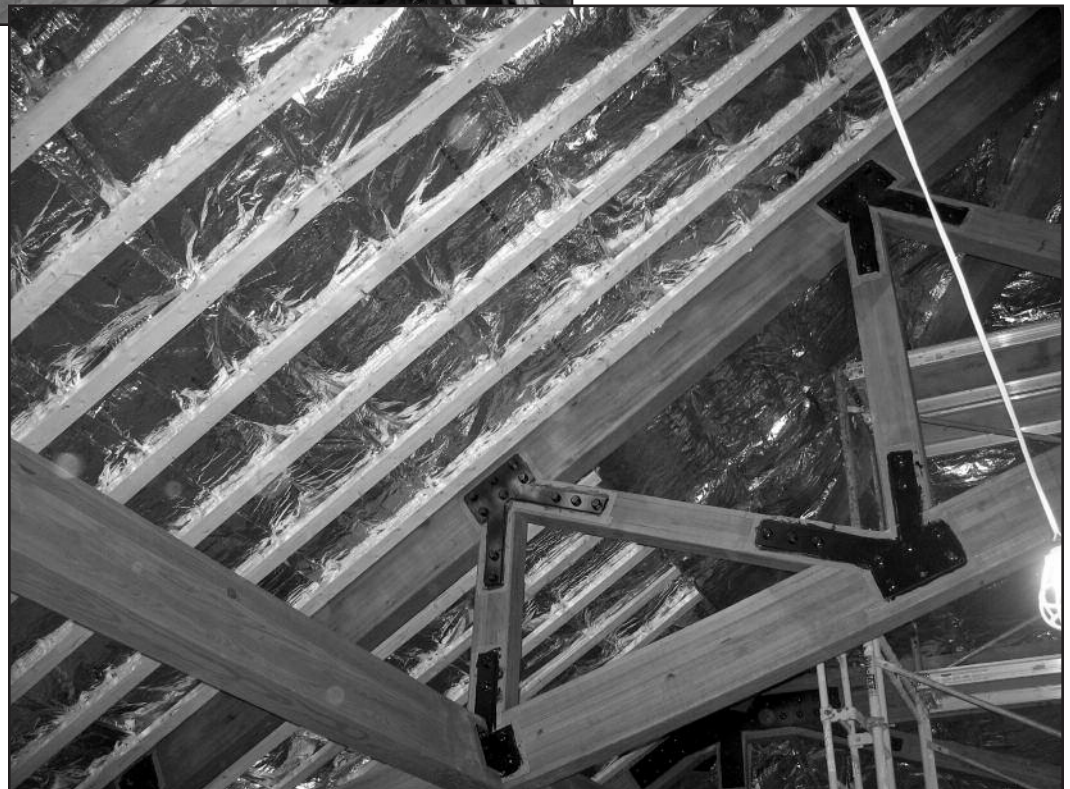
Figure 8 – Roof assembly under construction with Glu-Lam trusses and ceiling furring strips shown over FSK “vapor barrier.”
