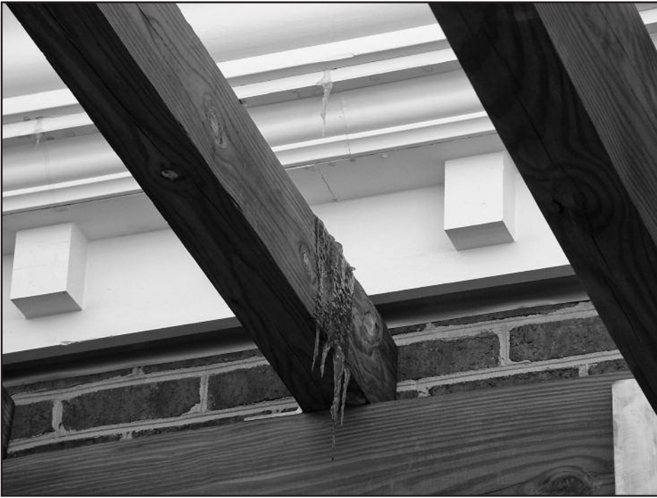
Figure 10 – Icicle formations where condensation was dripping from the pool-room eave.
