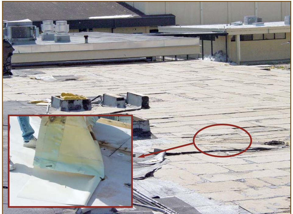
RIGID ROOF SYSTEM FAILURE
