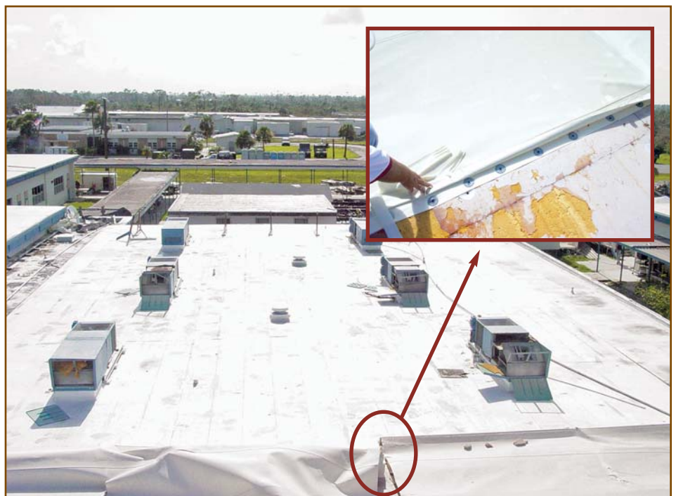
FLEXIBLE ROOF SYSTEM FAILURE
