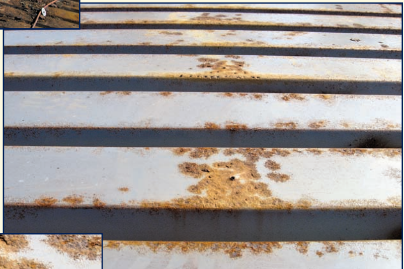
Photo 6 — Perhaps 60% to 70% of the deck area under the roof exposed by a full tear-off was found to be in this condition and treated with a rust inhibitor.
