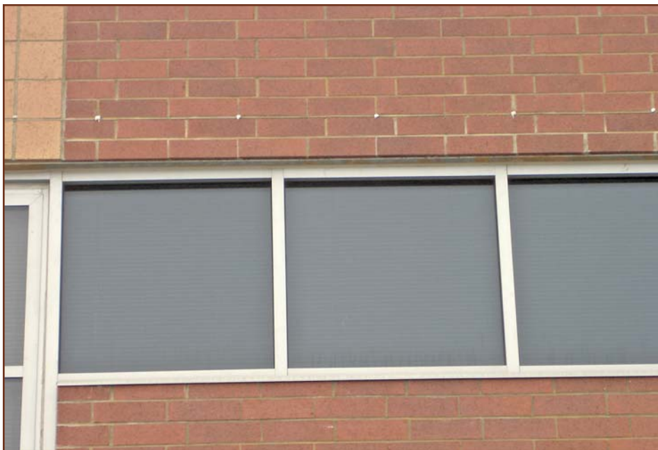
Figure 11 – Improperly located weeps.
