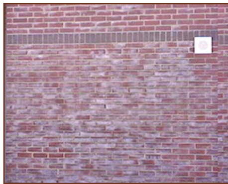
Figure 8A – Powdery efflorescence.
