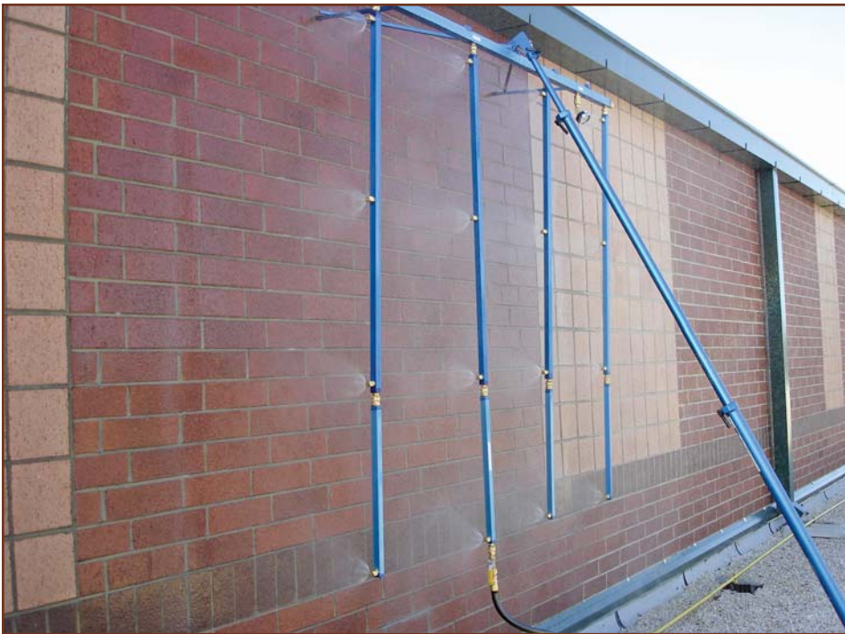
Figure 5 – Sheeting water created by water test.
