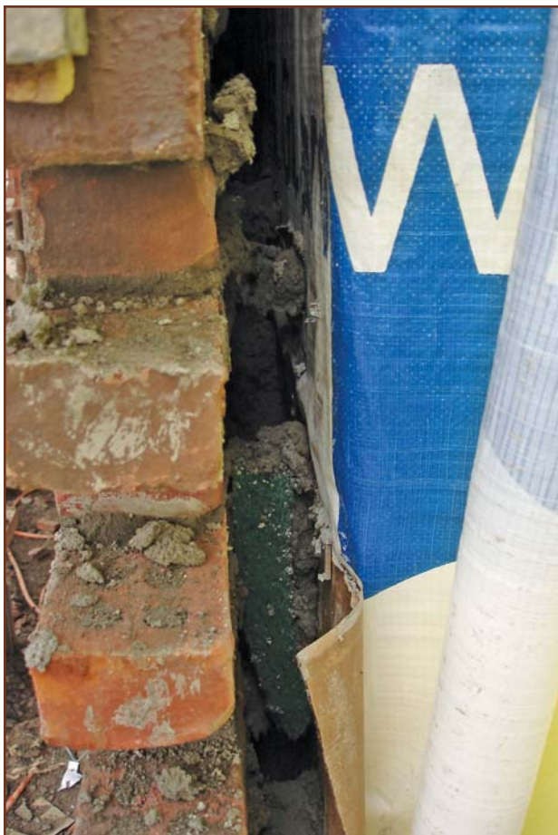
Figure 9 – Cavity impacted with mortar droppings.
