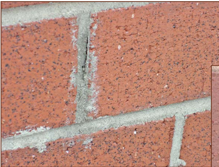
Figures 6A – Shrinkage cracks in mortar joints.
