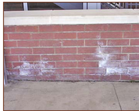
Figure 8B – Crystallized efflorescence.
