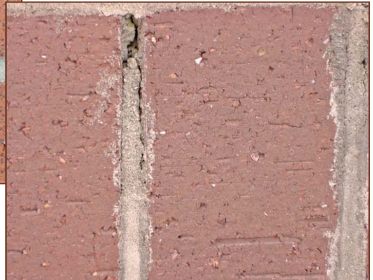
Figure 6B – Weak Bond in mortar joints.
