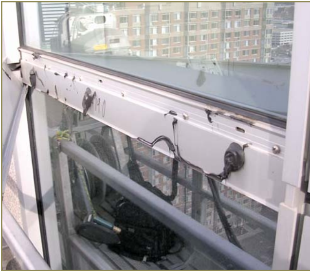
Photo 6 - Trim cover removed from curtain wall by hand with minimal effort.
