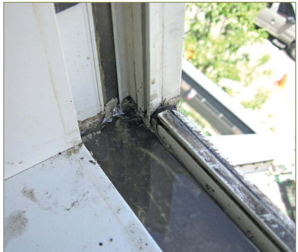
Photo 2 - Water ponding in curtain wall.
