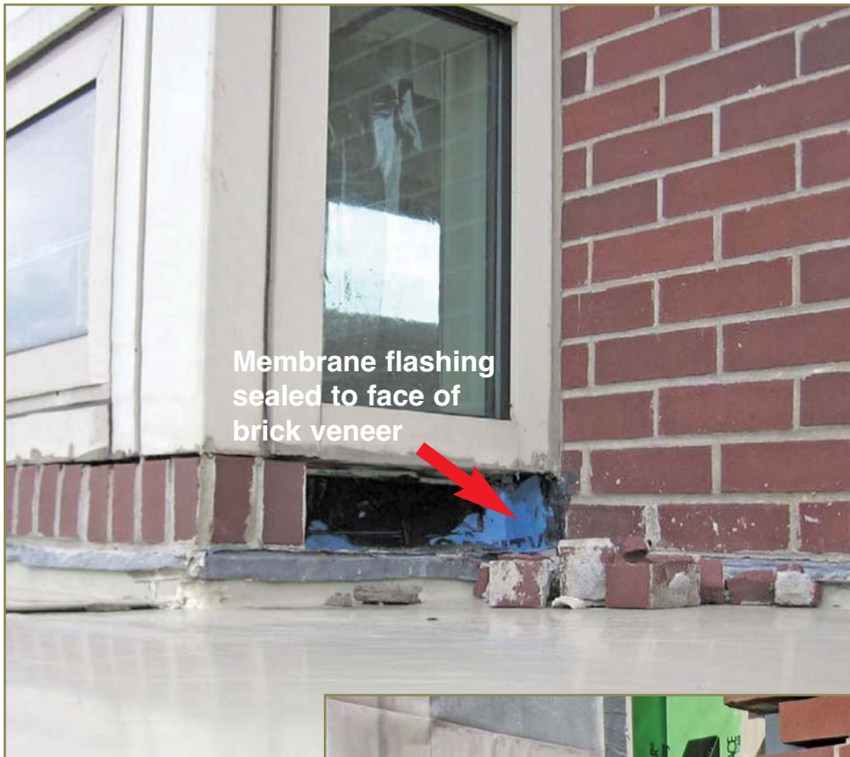
Photo 3 - curtain wall sill flashing not sealed to through-wall flashing.
