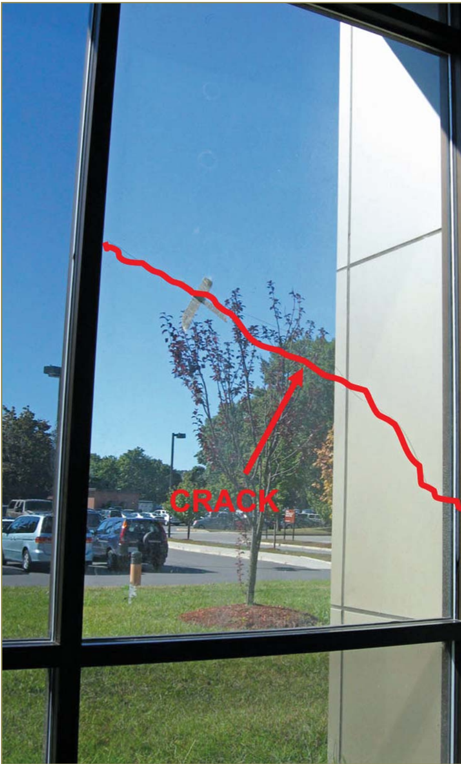
Photo 9 - Crack in IG unit.
