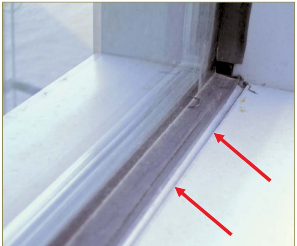
Photo 5 - Space between glazing gasket and trim cover.
