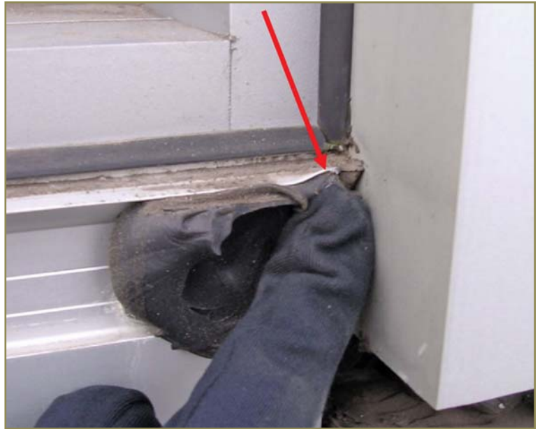
Photo 7 - Bent corner of pressure bar.
