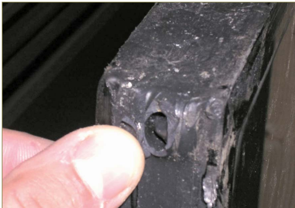
Photo 12 - Open blister in silicone secondary seal at the corner of an IG unit.
